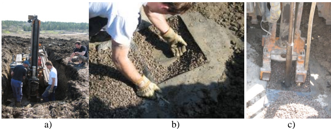
Figure 4 a) Excavation of the protection layer at the landfill site of Lilla Nyby, ca 6 month after closure, b) control of the drainage layer and c) sampling of fly ash stabilized sewage sludge layer.
