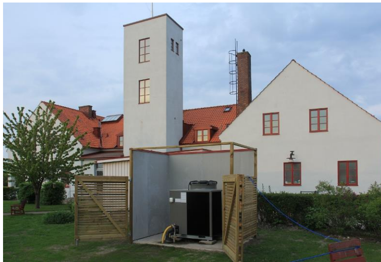
Figure 7. Heat pump location outside the day-care centre
