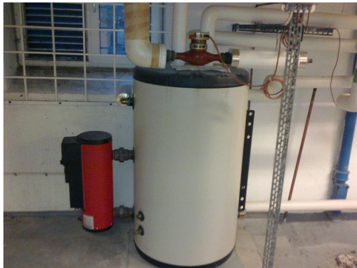
Figure 3. Hot water tank with electric heater (red)
