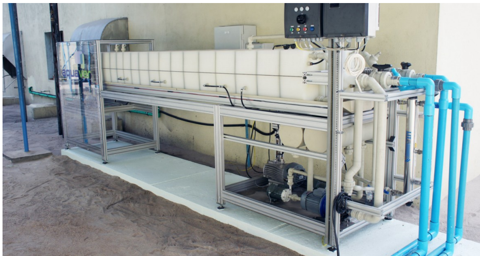
Figure 6. Memsys membrane distillation system integrated by Aquaver (Aquaver, 2015)
