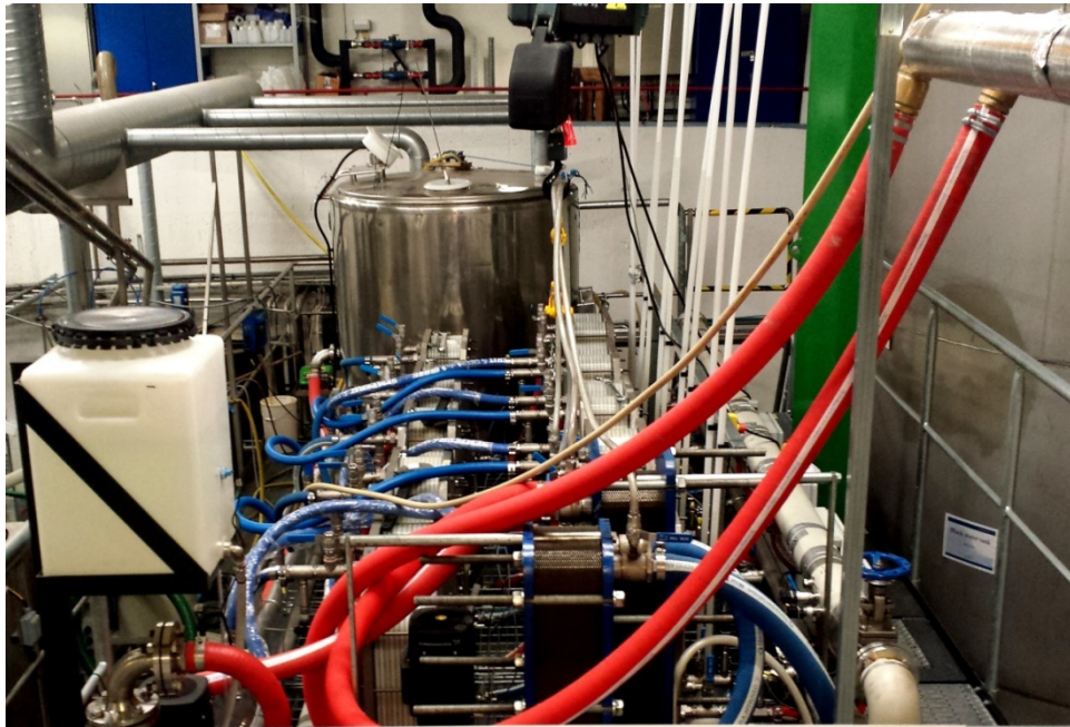
Figure 5. Xzero membrane distillation system at Hammarby Sjöstadswerk testing and demonstration facility.
