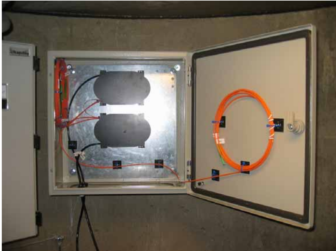
Figure 65 - Junction box installed in 2006.
