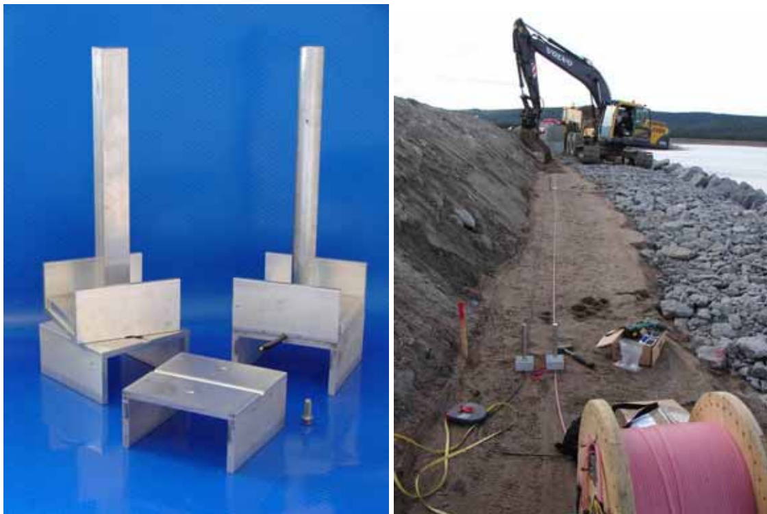
Figure 9 – Clamps used for the SMARTprofile cable and the DamSens cable, with additional surveying poles (left), and installation of the clamps at Seitevare dam.
