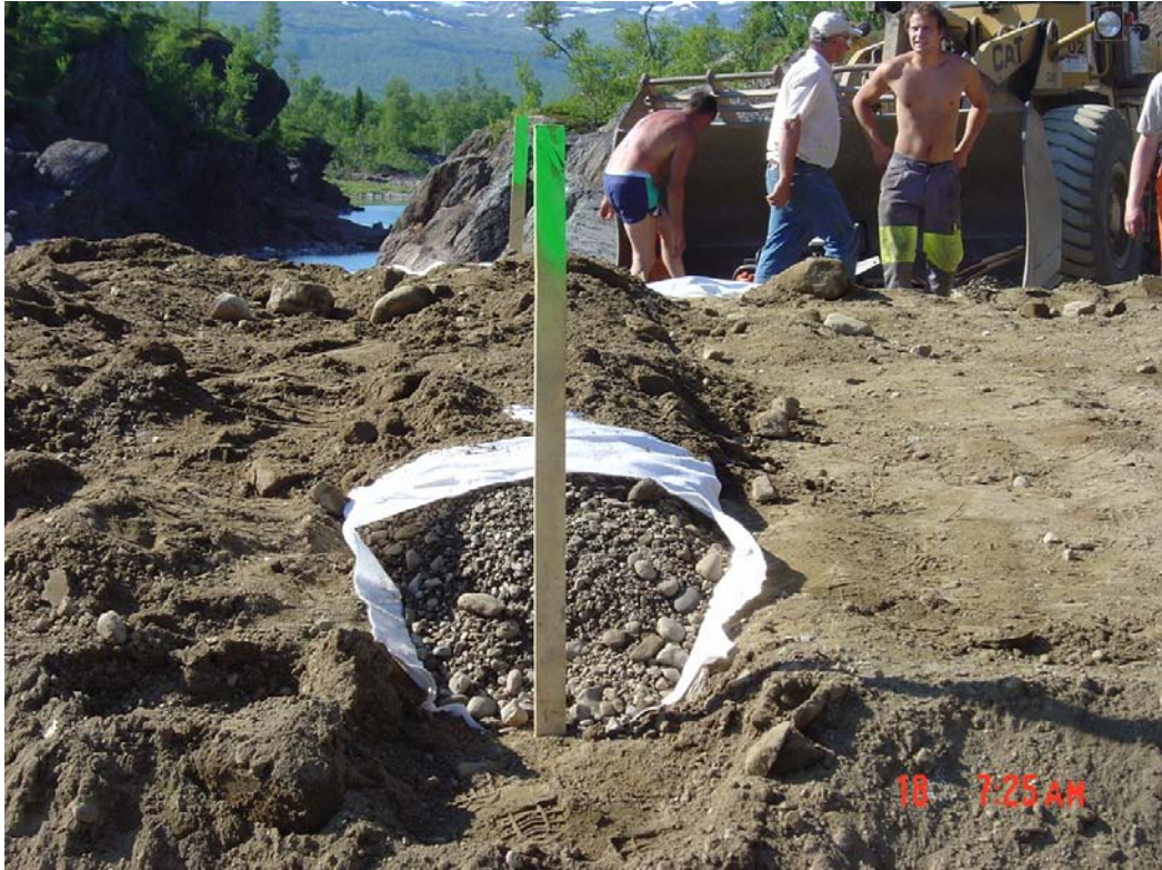
Figure 20 Defect A, the gravel in the defect is surrounded of filter fabric before the placing of the moraine continued
