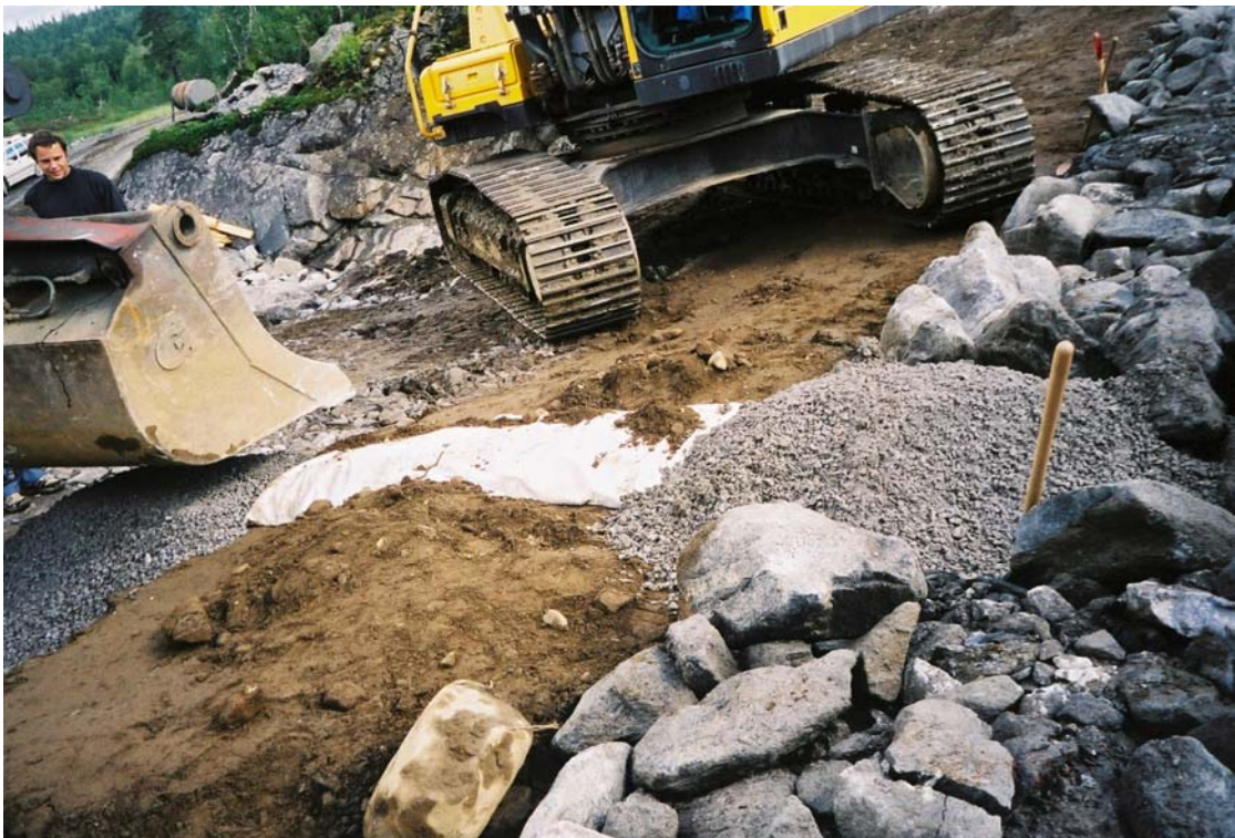
Figure 23 Defect C, filter fabric surrounds the gravel and filter has been placed to connect the material in the defect to the rock fill in the shoulders of the embankment.
