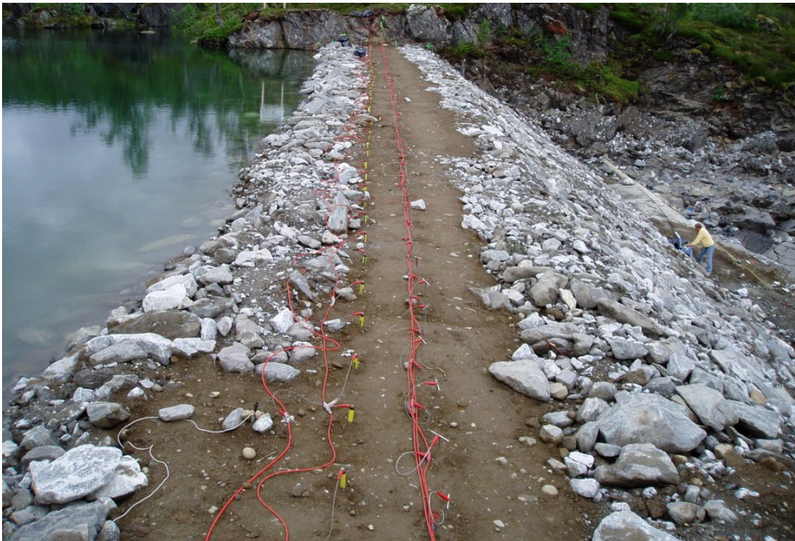
Figure 9-1 Electrode layout along the dam crest at the Røsvatn test embankment dam, with non-polarising Cu-CuSo 4 electrodes (for SP) to the left and stainless steel electrodes (for resistivity-IP) to the right.
