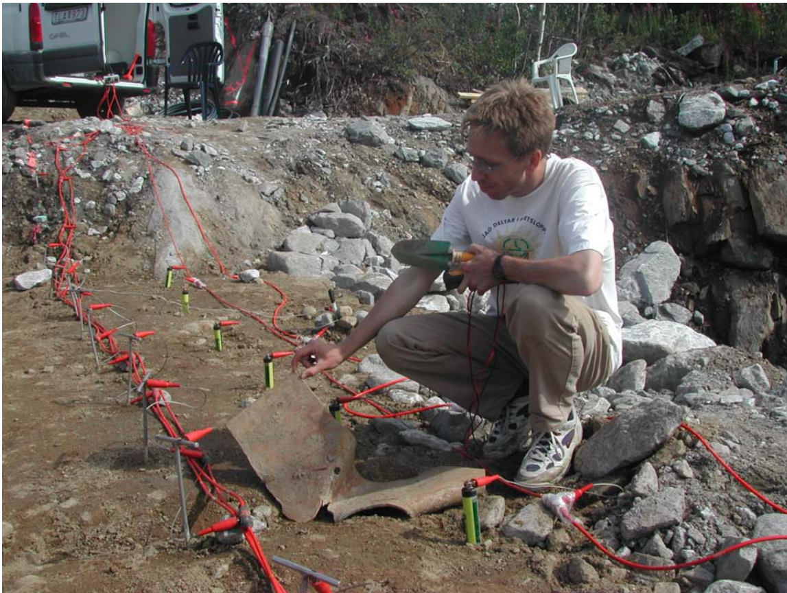
Figure 11-1 Steel plate found on the crest.
