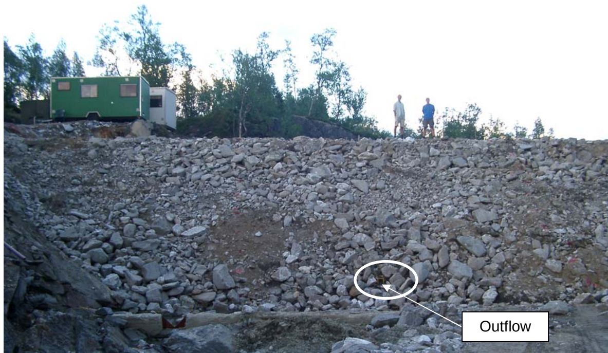
Figure 9 Observed outflow at sec 27m, about 1m above the concrete sill. The high amount of fines in the support fill can also be seen.
