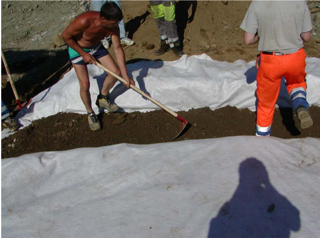
Figure 22 Defect B, the gravel in the defect is placed and surrounded by filter fabric
