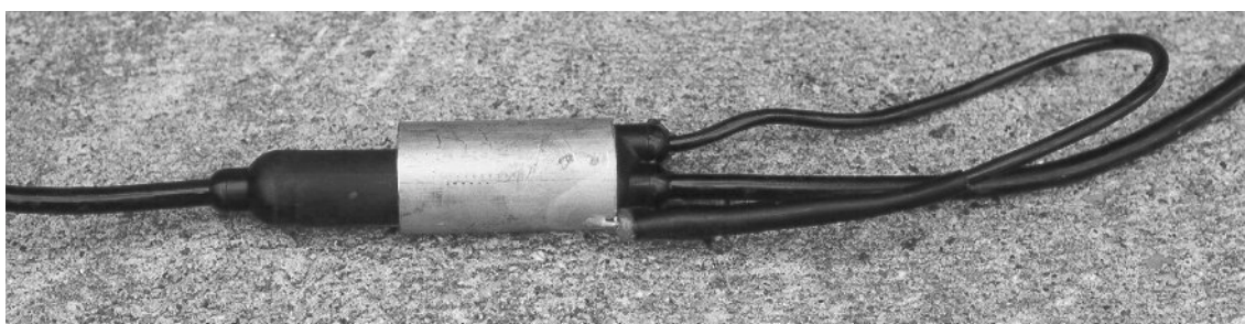
Figure 7 Electrode mounted on multi-core cable used on the upstream side.
