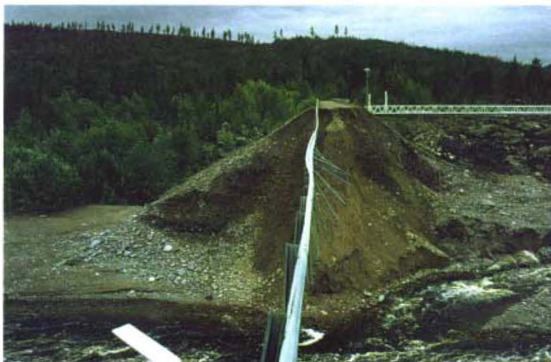
Figure 3.9. During the rainy autumn of 1985, the groundwater level in Dalarna had risen to above the normal level. When this was later followed by a particularly heavy and long-lasting rainstorm, and at the same time one of the spillways in the Noppikoski Dam failed to open, the earthfill dam was overtopped with a resulting dam failure. This caused the 1 Mm 3 reservoir to be emptied in less than an hour. The flood wave caused damage over an area along 20–30 km of the river.
