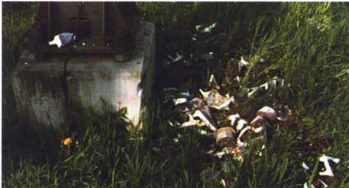
Figure 6.2. A L2-phase surge arrester has exploded when struck by lightning. The photograph is intended to point out the risk of lightning causing power station outage, which means that the turbine water has to be released through the spillways. It is, of course, necessary in this context to make sure that the spillway function will not also be damaged on the same occasion, or in other words that the power supply and control equipment are fitted with a good lightning protection system.
