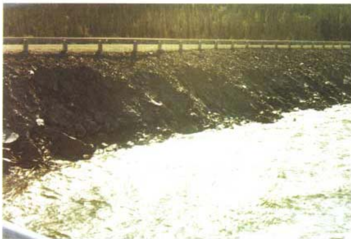
Figure 4.2. Damaged erosion protection on the upstream shoulder.
