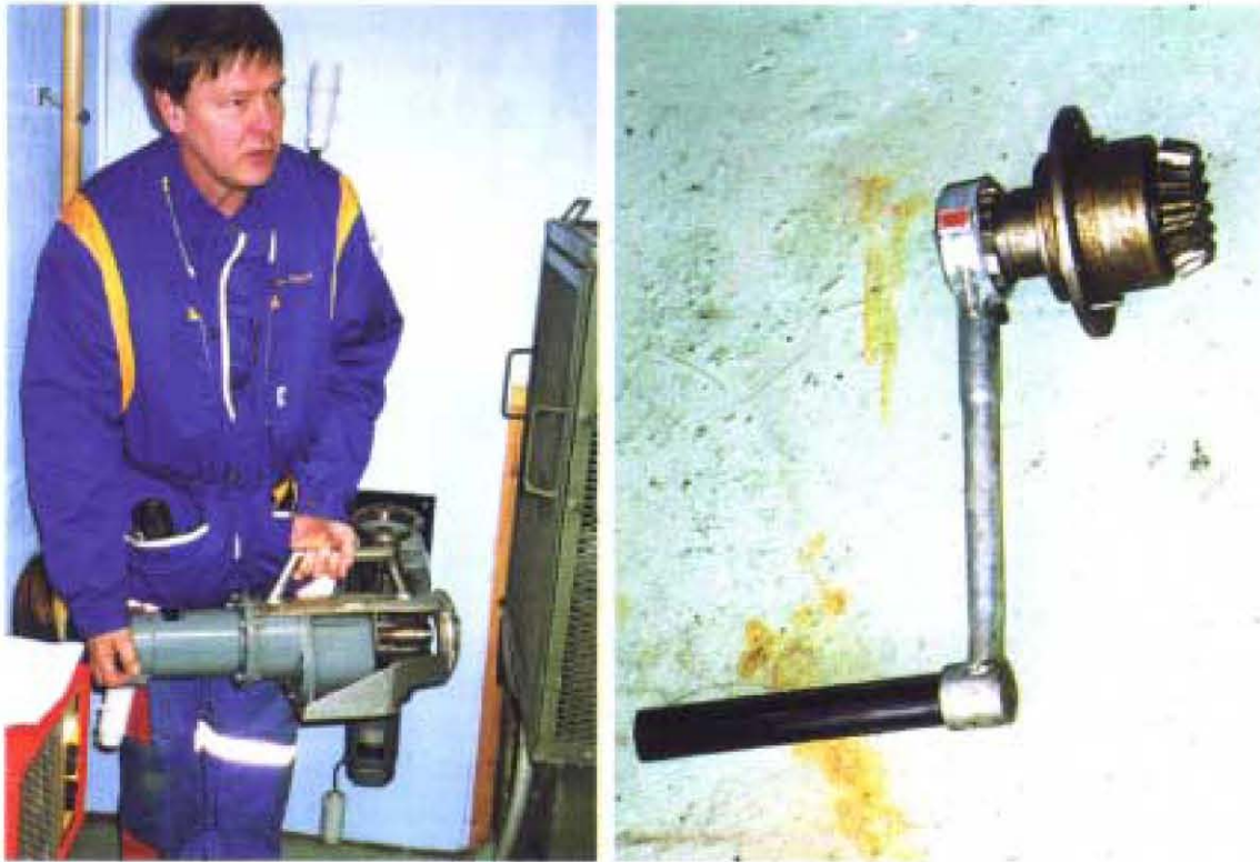
Figure 6.3. The machinery of spillway gates often has a connection for a crank in order to make it possible to open the gate if both the power and back-up power have failed. It is recommended to replace the handle with an electric motor, which can be powered from the electric system of a car or an equivalent system.
