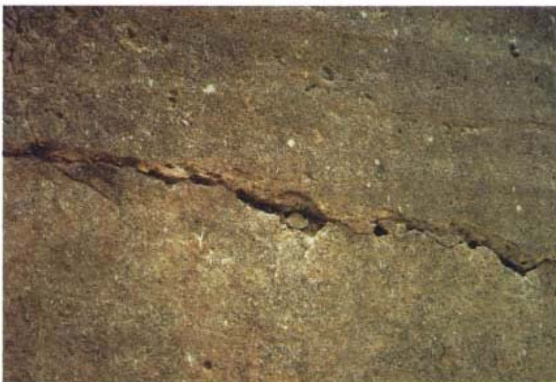
Figure 8.2. Porous concrete on the surface of a canal wall at a fracture.
