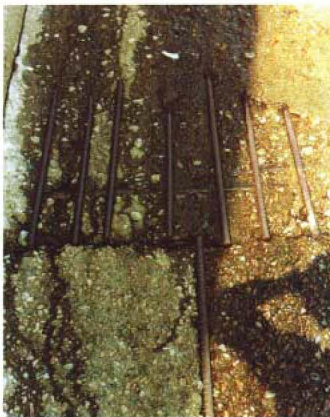
Figure 5.2. Damaged concrete in a spillway.
