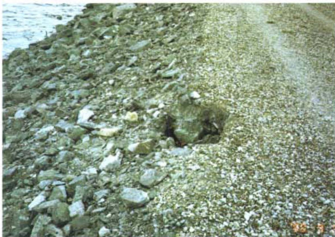
Figure 4.8. Erosion channel at toe of sheet piling (above) and sinkhole in crest of dam (below).
