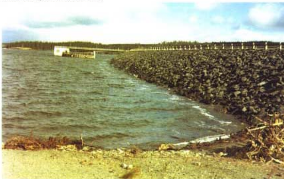
Figure 4.5. Erosion protection with a surface layer of randomly-laid boulders.
