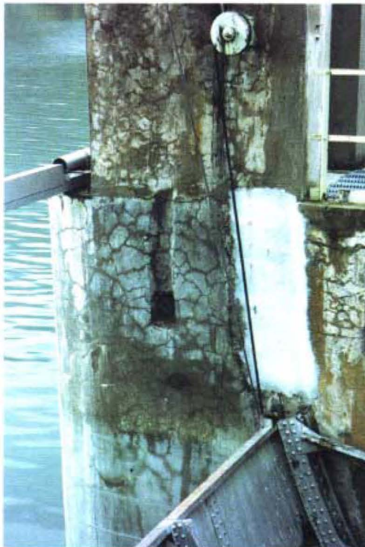
Figure 8.5. Typical damage in concrete with alkali-reactive aggregates.
