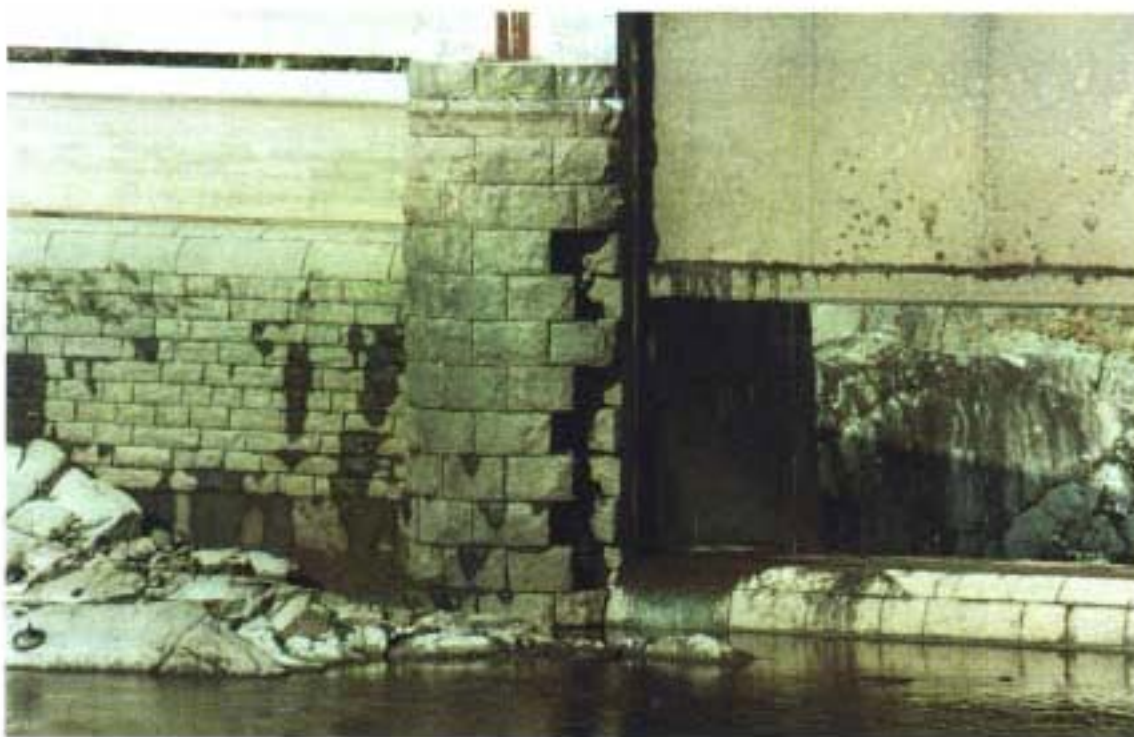
Figure 6.1. Spillway columns with stones that have disappeared.
