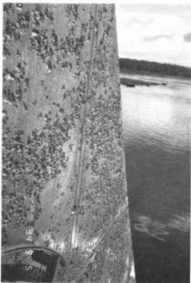
Figure 8.3. Flaking of material on the surface of a spillway column.
