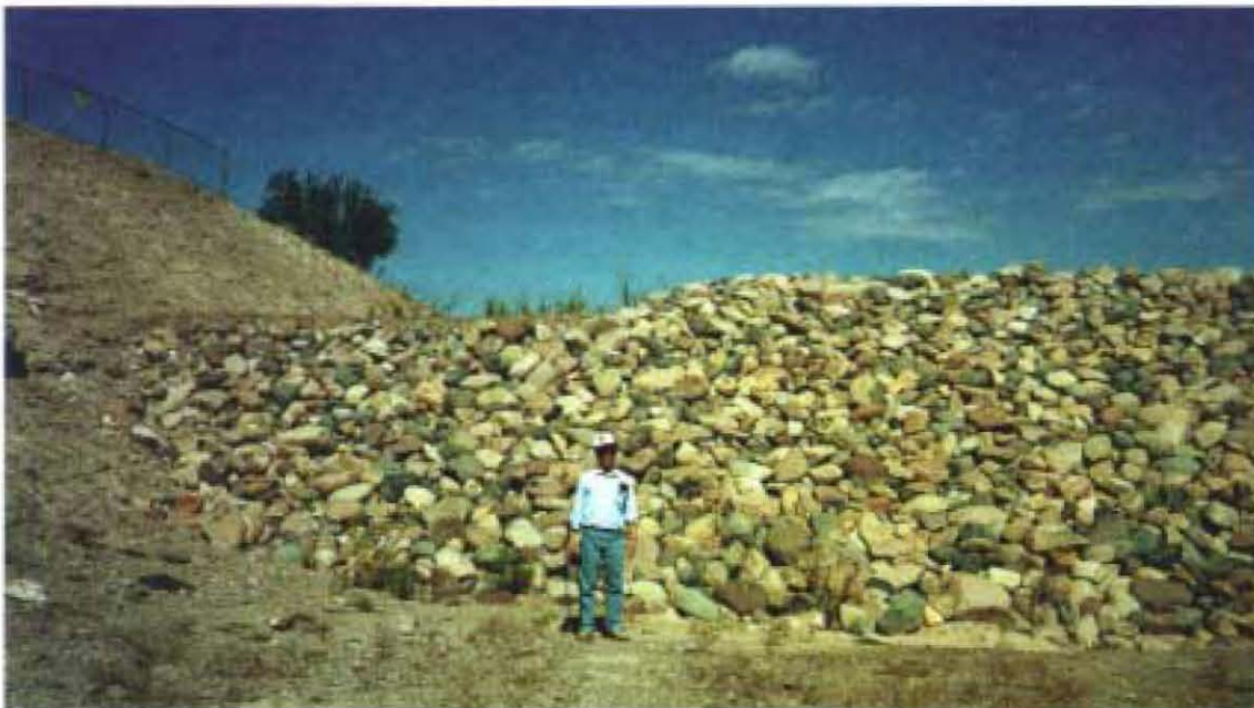
Figure 6.10. An erodible section of dam (fuse-plug) in the USA (left side somewhat lower to facilitate initiation).
