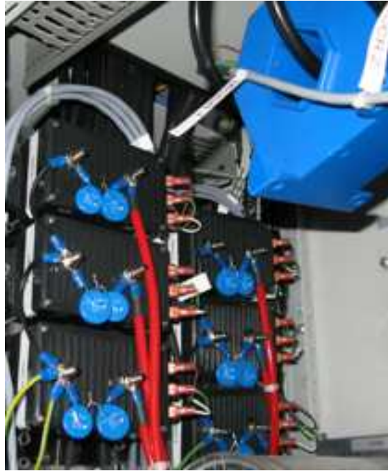
Figure 7.2: Voltage sensors measuring the voltages on the rotor as well as on the 480 V side of the wind turbine transformer.
