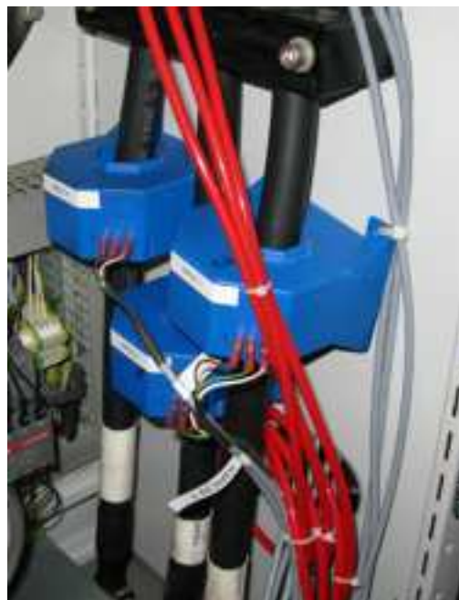
Figure 7.3: Grid converter current measurement.
