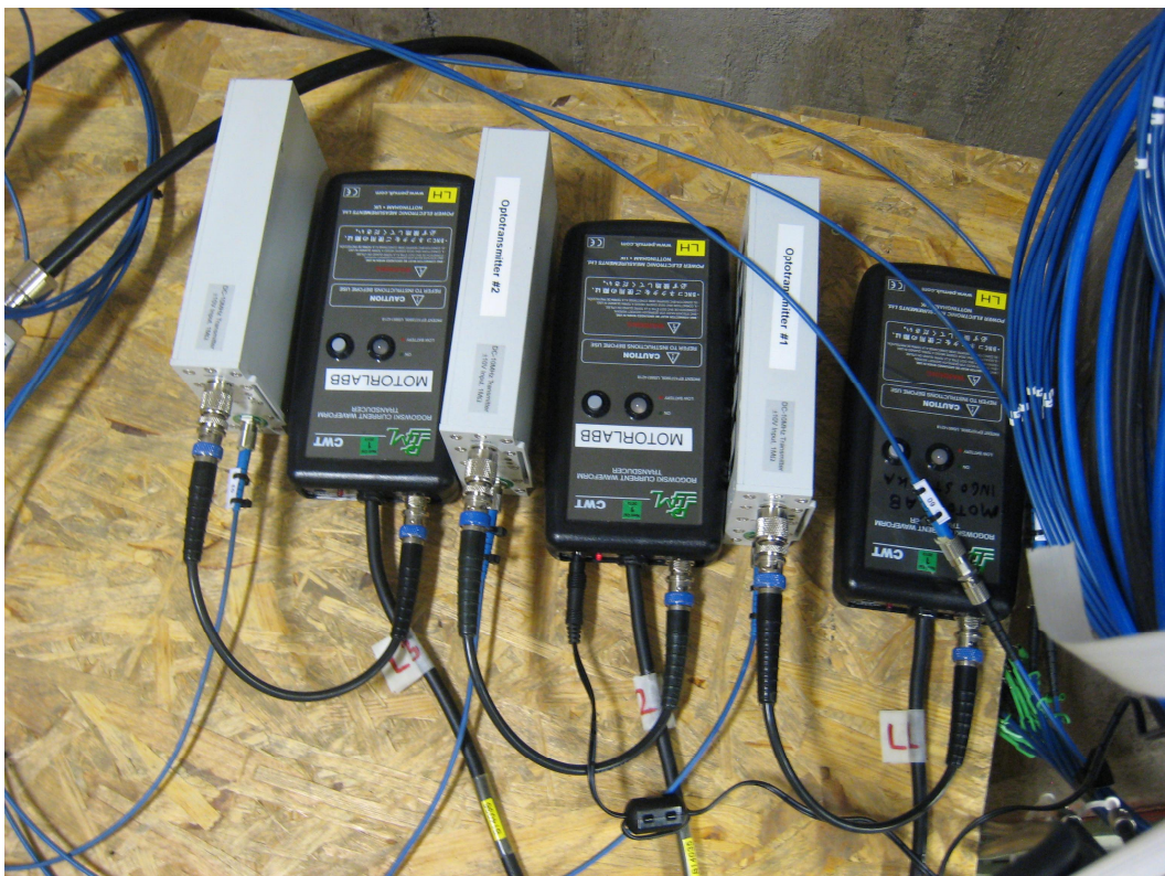
Figure 91 Measurement Data transmitters and battery chargers
