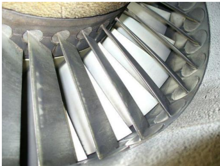
Figure 20. Compressor IGV and rotor 1 after 28,000 hours of operation with HEPA-level (courtesy of VGB)
