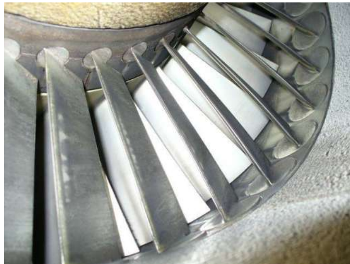
Figure 7-4. Compressor IGV and rotor 1 after 28,000 hours of operation with HEPA-level (courtesy of VGB)
