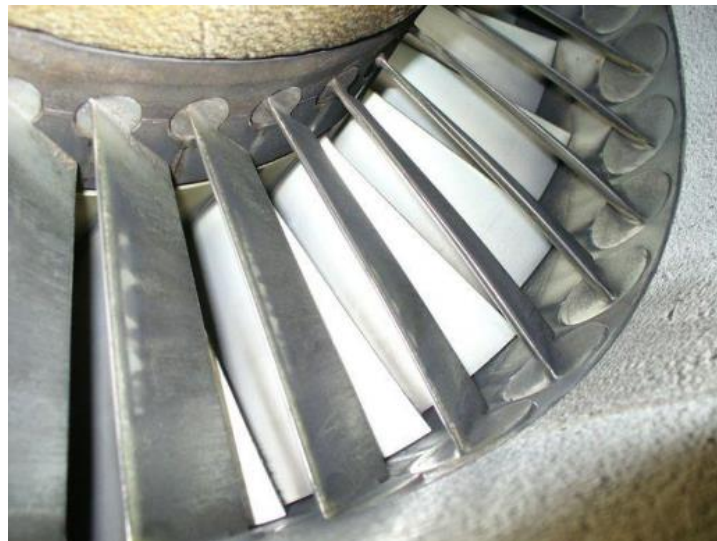
Figure 7-6. Compressor IGV and rotor 1 after 28,000 hours of operation with HEPA-level (courtesy of VGB)
