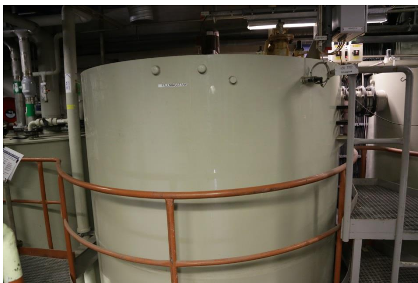
Figure 3. A container made of polypropylene used in the water purification process in a flue gas facility.
