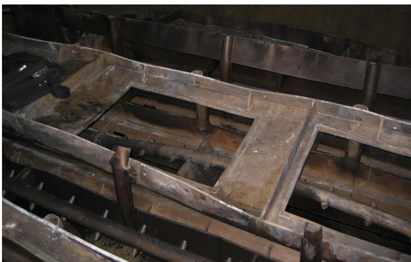
Figure 1. Typical example of distortion of PP components in a flue gas scrubber due to thermal expansion and contraction of the material.
