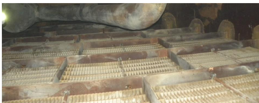
Figure 2. One example of the use of PP for droplet separators in flue gas scrubber in a waste incineration plant.
