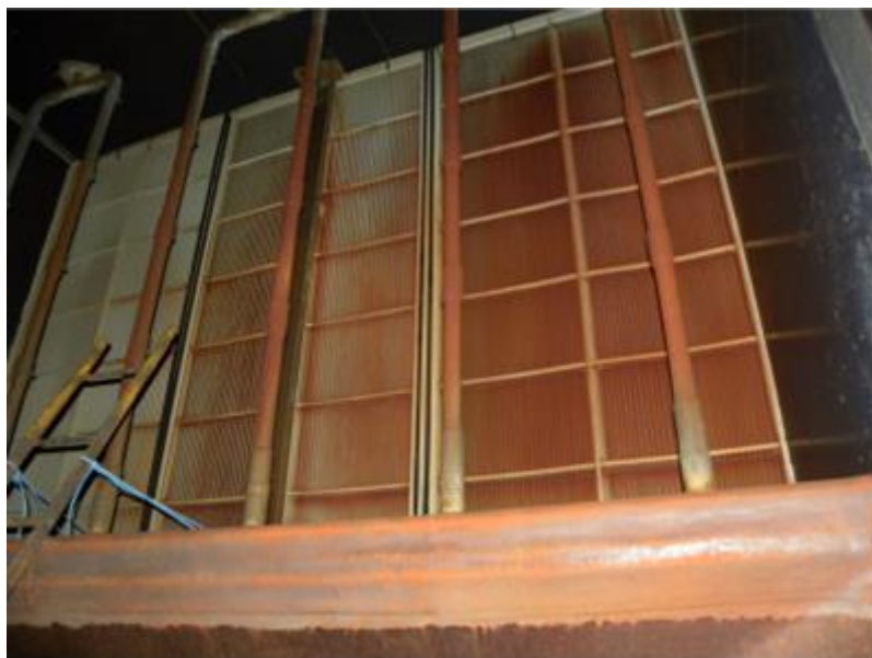
Figure 4. Droplet separators in the scrubber in a waste incineration plant which had an OIT of 0 minutes at the surface after only 6 months of service but have still lasted for many years without becoming brittle from oxidation.
