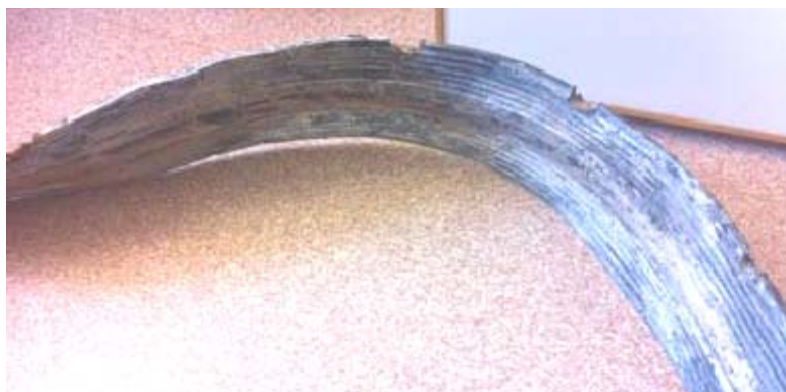
Fig. 4. Sealing strip from Ringhals after 30 years of operation [ELFORSK2013].
