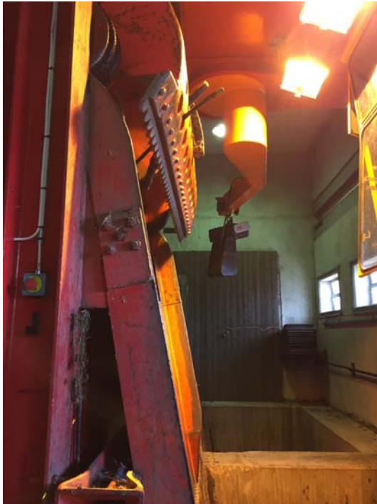
Figure 4. Scrape for removing trash and ice from the intake gates.
