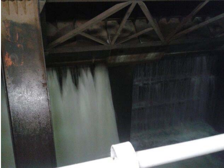
Figure 3. Frazil ice blockage of a water intake at Hjäлта hydro power plant.
