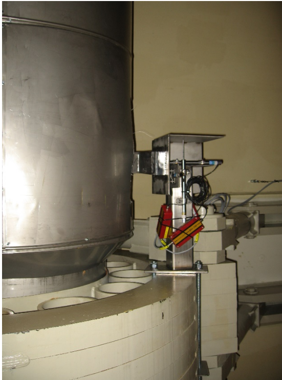
Figure 3 Axial and lateral mechanical LVDT sensors mounted on steam pipe. Source "delivered from RAB".
