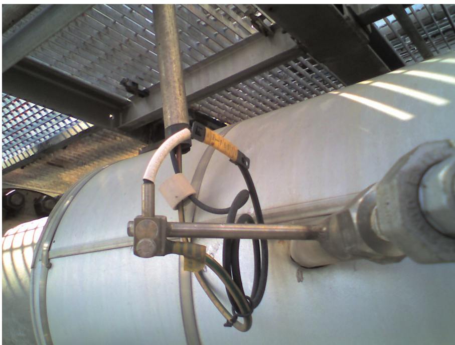
Figure 17 AE-probe mounted on a hot cracker tube pipe. The probe enters the main pipe in 30 degrees and registers the change in the process. Source “example figure from non-nuclear industry”.
