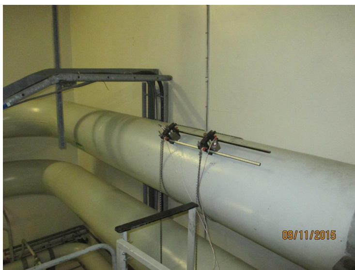
Figure 16 Ultrasonic flow meter attached by chains. Source “delivered from participating plants”.
