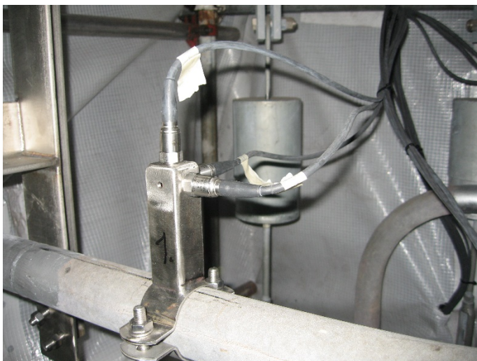
Figure 4 Accelerometers in three perpendicular directions mounted on a U-clamp on a pipe without isolation. Source "delivered from RAB".
