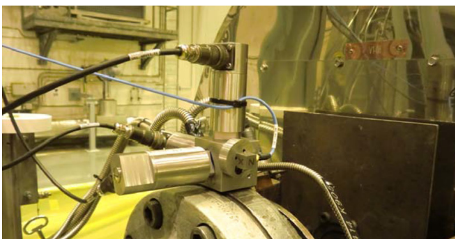
Figure 31 Example of mounting of accelerometer and velocity transducer on a high pressure steam emergency safety valve housing. Source “delivered from participating plants”.
