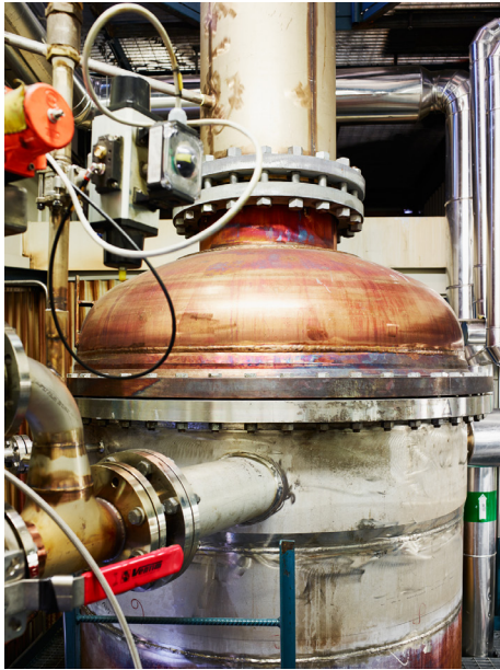
Figure 2: The primary gasifier in Hortlax with its two fuel inlets.
