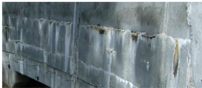
Figure 3.1: Efflorescence stains at the concrete surface due to cracking.
