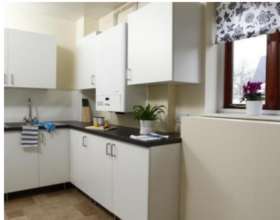
Combined Heat & Power (CHP)
