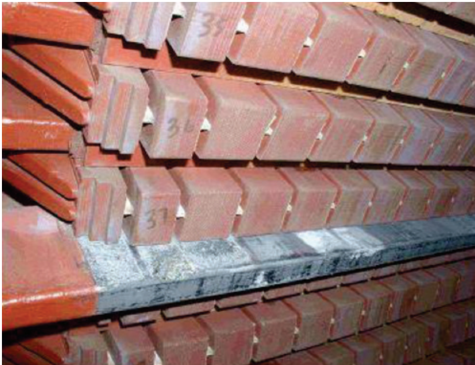
Figure 55. Vibration fretting of main insulation in slot parts
