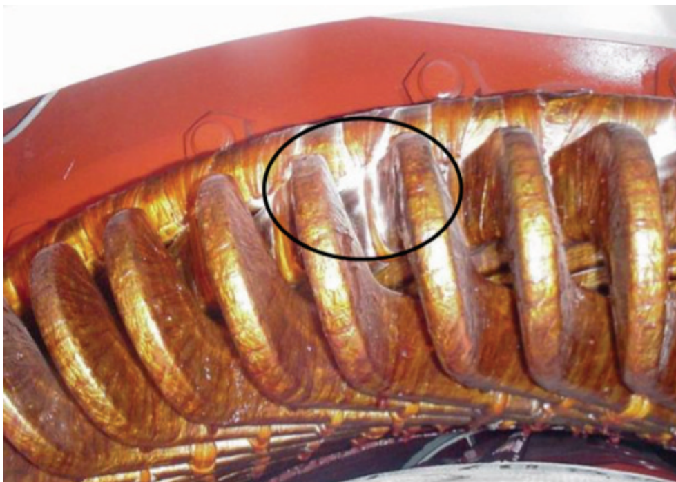
Figure 50. Fretting in tangential blocking between bar knuckles
