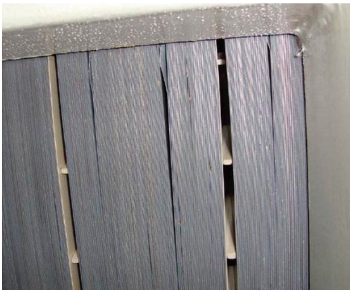
Figure 64. Lack of pressure in the core back
