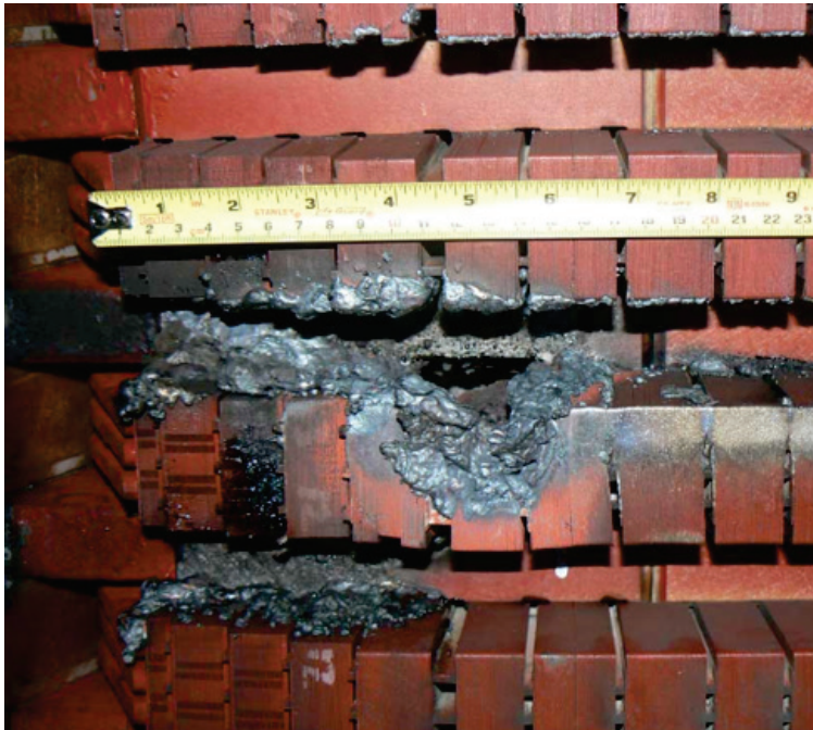
Figure 62. Partial meltdown of the core air gap surface.
