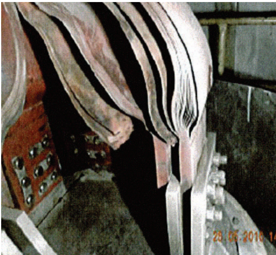
Figure 60. Partly broken braid between winding and bus bar
