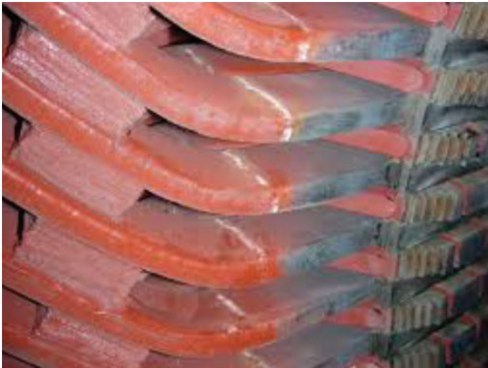
Figure 57. Broken connection between corona protection at slot portion and end-winding
