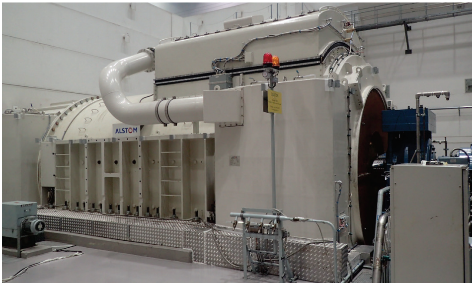
Figure 90. Generator in Olkiluoto 1 and 2
