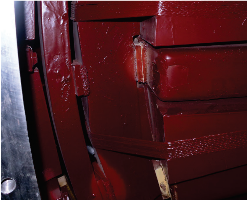
Figure 83. Cracks and fretting powder in bracing outside knuckles
