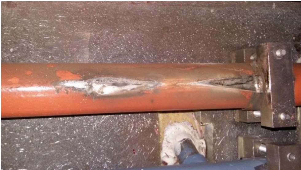
Figure 86. Wear marks on manifold
