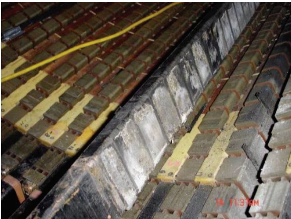
Figure 56. Vibration sparking on bar at neutral of the winding
