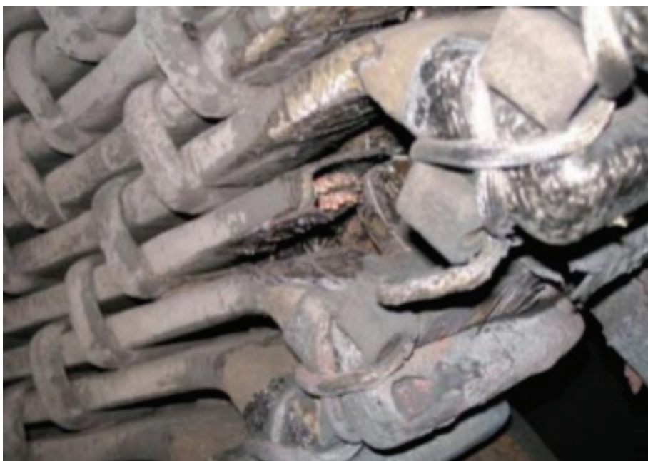
Figure 58. Broken connection between end-winding and round connection, caused by vibration
