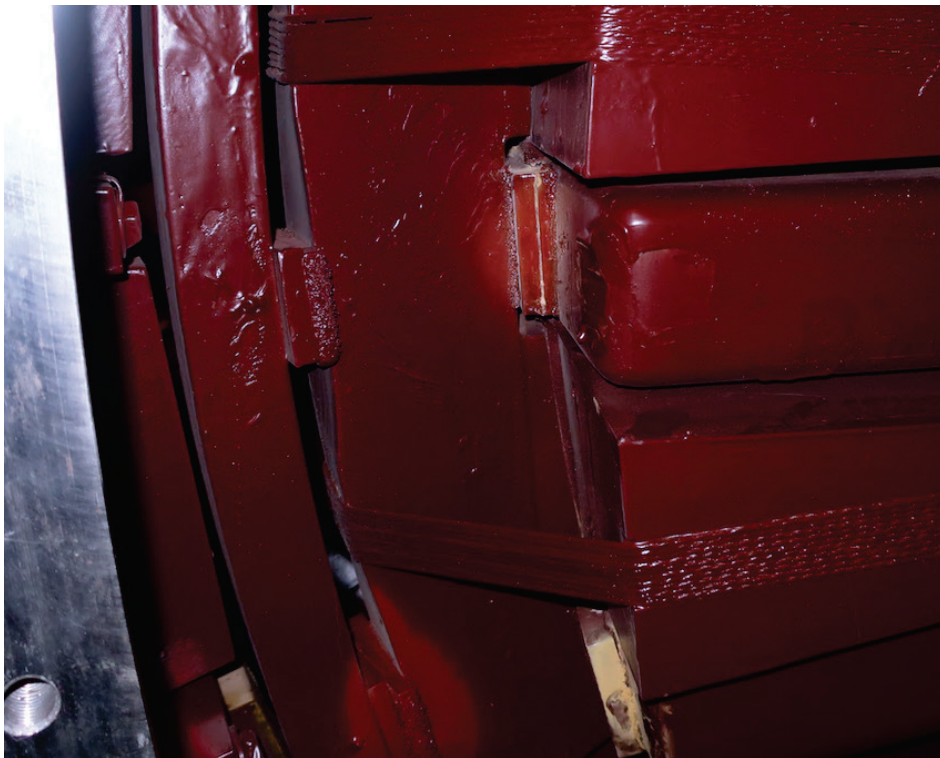
Figure 51. Tangential blocking with degenerated prestress forces causing cracks and abrasion dust
