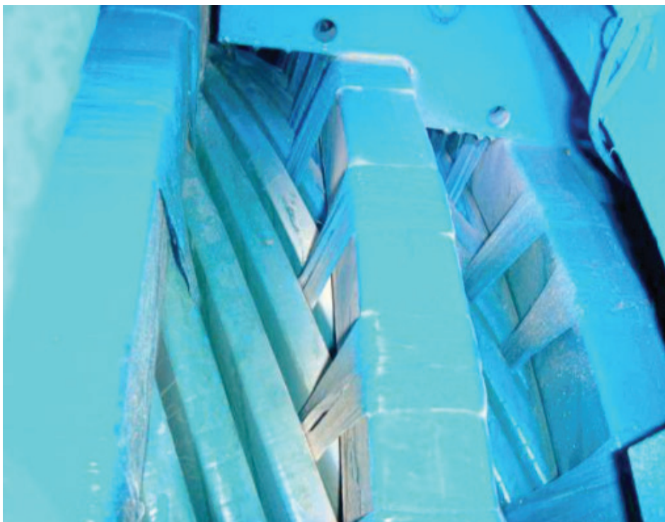
Figure 52. Lost prestress tension in fixation bandage between bars and support rings. In stator of resin ring type se figure 28
