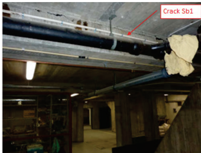
Figure 5-12 Crack (joint) Sb1 under bjl +83,70.
