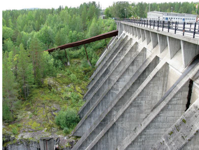
Figure 94 The downstream side of the regulating dam, before any measures were taken.
