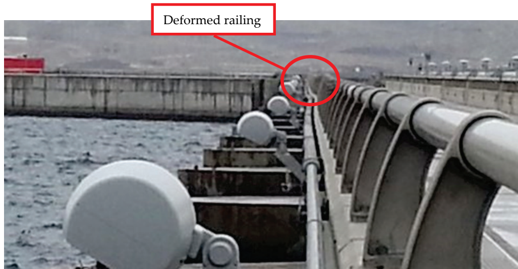
Figure 4-1 Deformed railing on the dam crest, Wanapum Dam.
