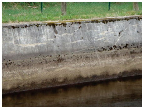
c) Internal frost damage above the water-line, as well as surface damage and leaching under water-line in a guide wall
