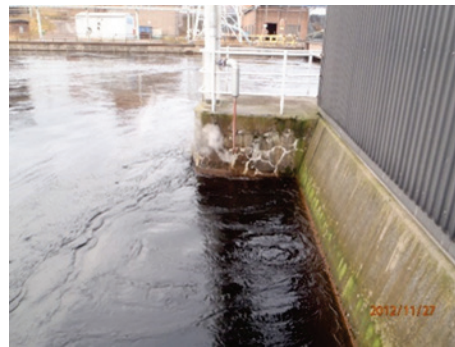
b) Internal frost damage at the intake of a power plant.
