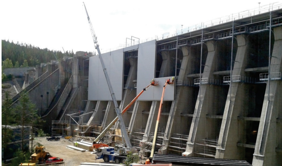
Figure 4-7 Assembly of an insulation wall to decrease thermal movements on a buttress dam
