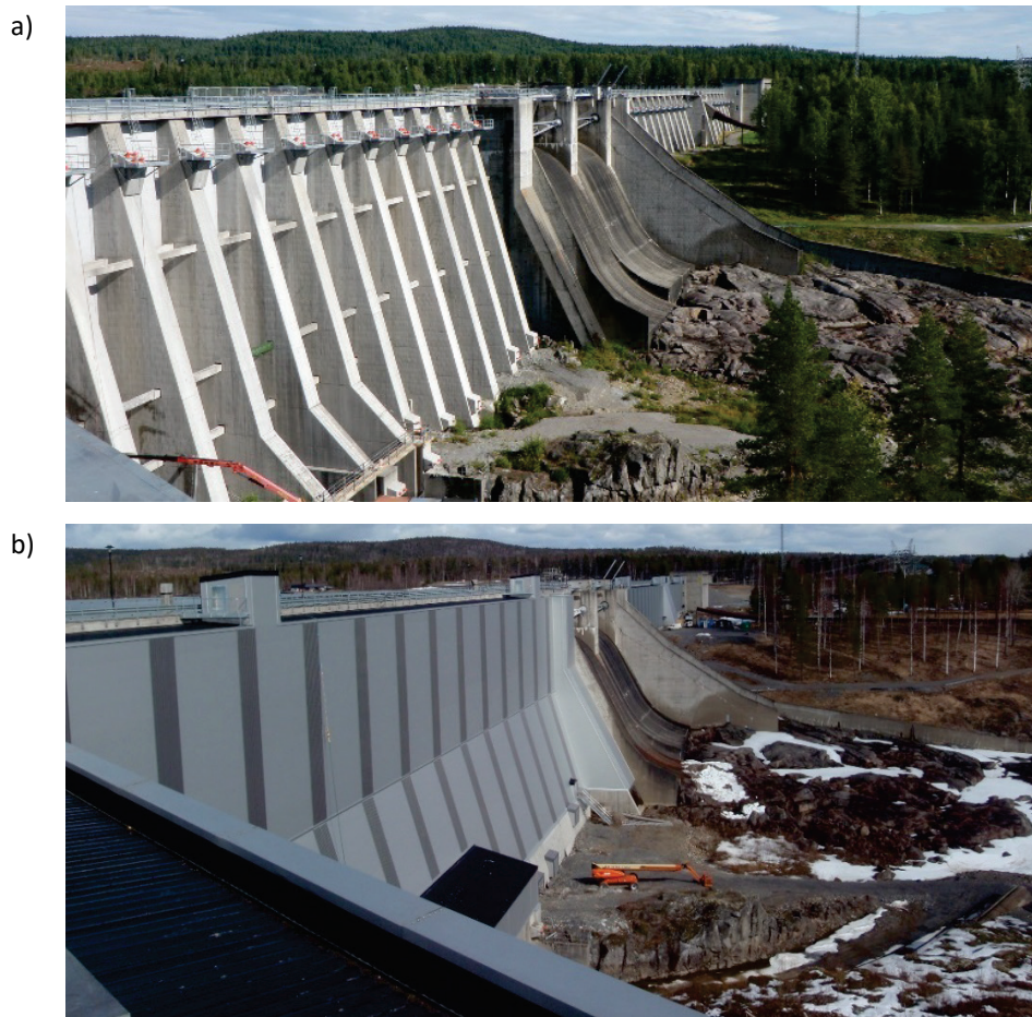
Figure 5-73 a) Photo with the old insulation wall (Foto: Christer Vredin/Sweco), b) photo with the new insulation wall (Photo: Maria Marklund/Sweco)
