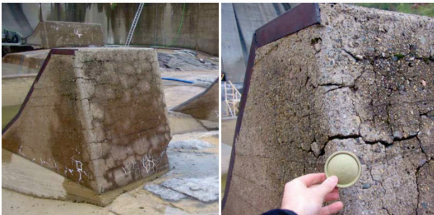
Figure 2-19 – Flow splitter damaged by ASR [23].
