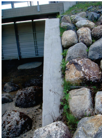
Figure 2-21 – Structure damaged by ASR with a cracking plane parallel to the main reinforcement.
