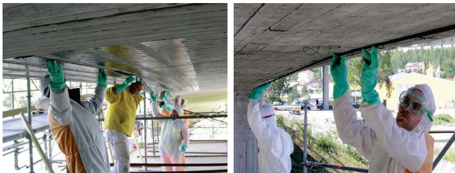
Figure 4-19 Reinforcement in bending with carbon fibre composite. Laminate (left) and anchors (right). [80].
