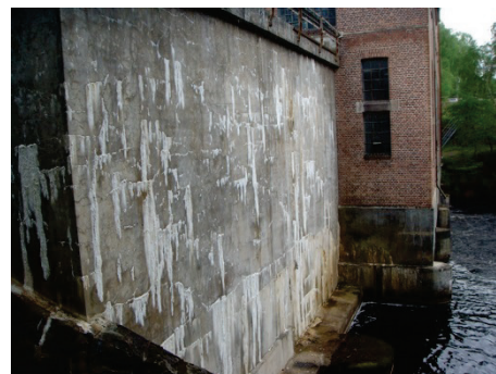
b) Leaching through cracks is common in old structures.
