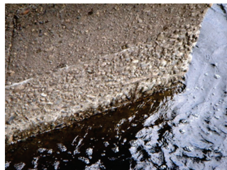
b) Surface peeling at the water-line, [11].
