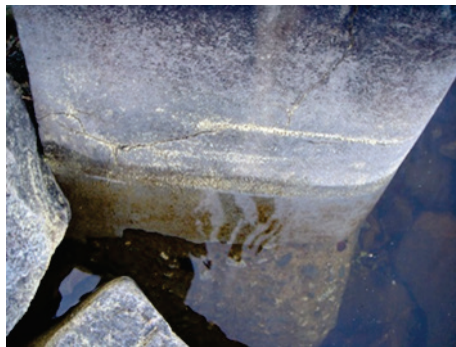
a) Internal frost damage of a structural part above the water-line
