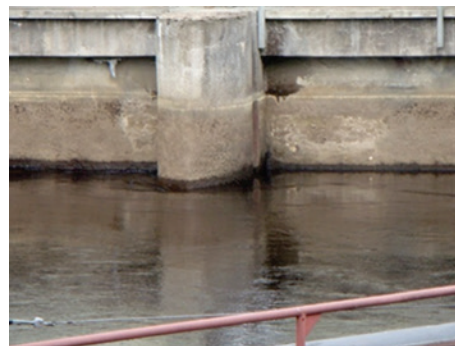
d) Damages like in picture c) but at the intake
