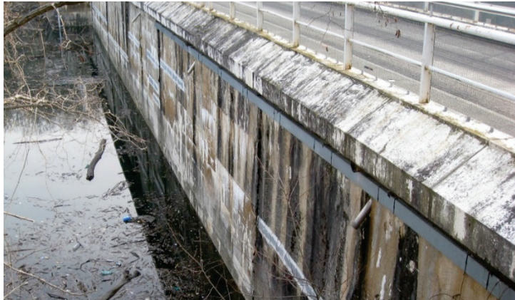
Figure 4-9 Sealing of cracks with strips of sealing material on concrete dam of the massive type
