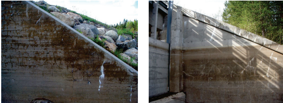
Figure 2-18 – Structure damaged by ASR with a varying crack pattern.
