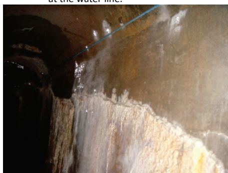
c) Leaching through a crack, which most likely occurred due to prevented thermal movement.
