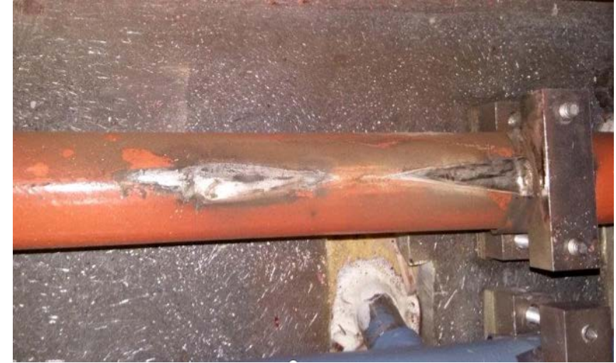
Wear marks on manifold
