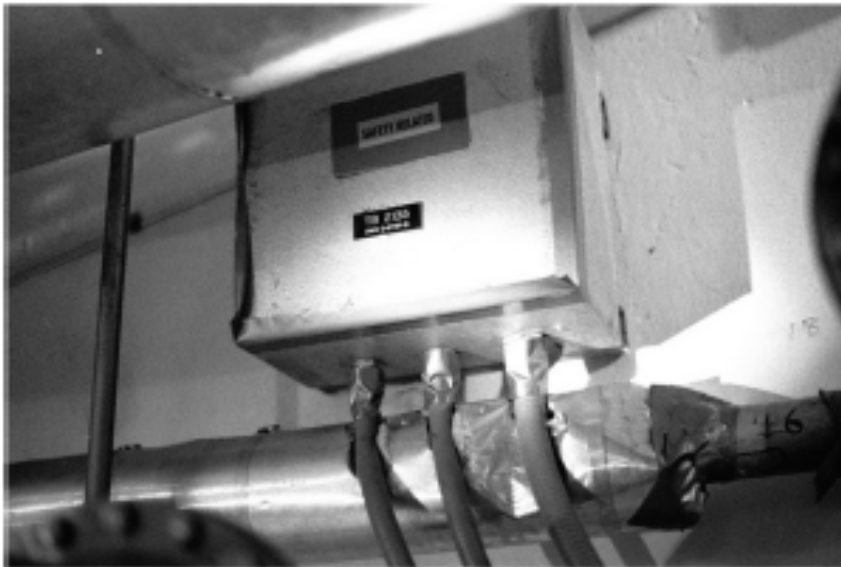
Displaced thermal insulation on valve operator
