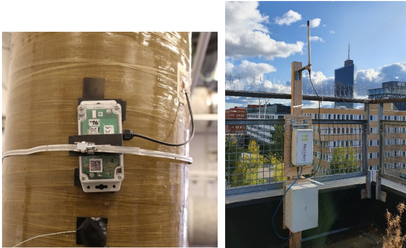
Figure A2: The sensor housing containing the radio sensor with a connected piezo crystal mounted on an FRP-construction. Figure A3: The gateway installed on the roof of the building communicating with the installed sensors and enable the data online.
