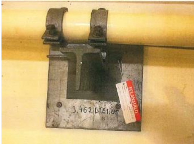
462L151/U5 Vibrations (loose expanders)
