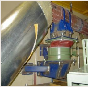
VD (VES type) at the Feed-water piping in a high radiation zone
