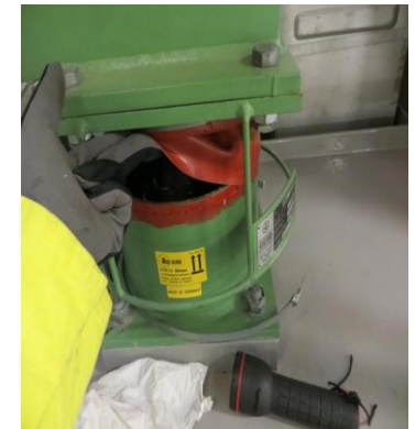
Viscodamper with broken sleeve
