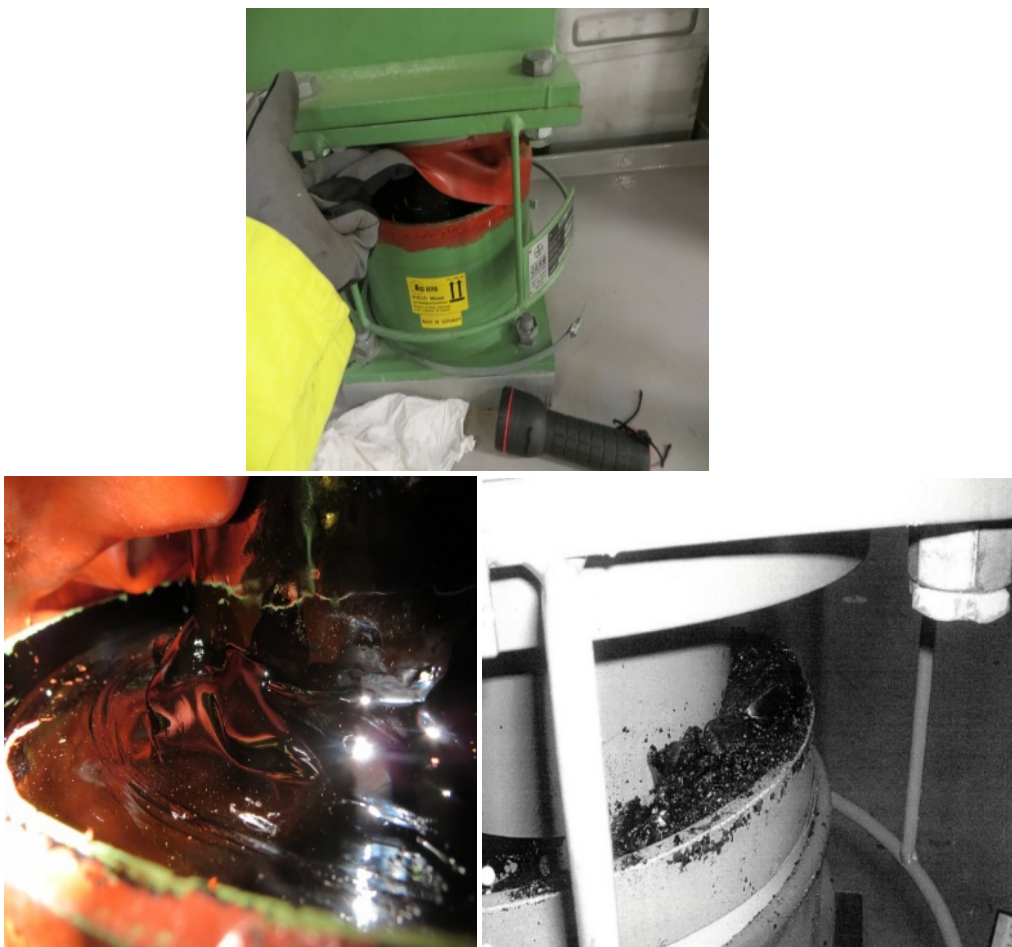
Figure 42: Example of broken sleeve and cracked fluid of viscous damper.
