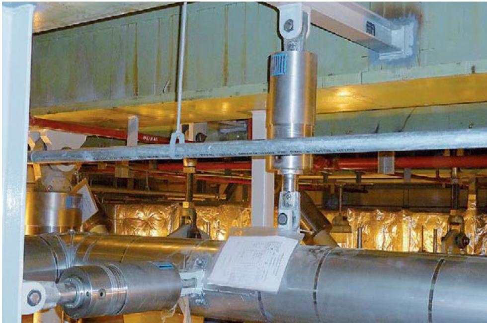
Figure 11: Pipe system secured with snubbers
