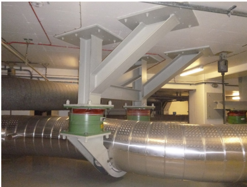
Figure 33: Example of a number of viscous dampers and how they are connected to supporting construction.
