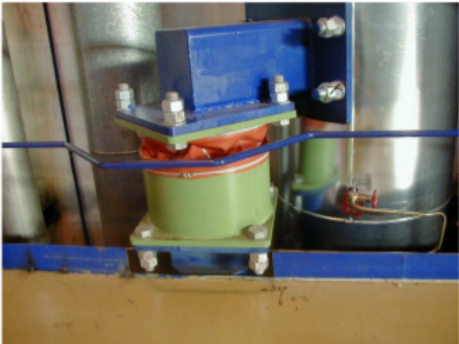
Figure 60: VD damper installed at the RA11 in Turbine Hall with damper piston at the piping and the housing at the TH floor.
