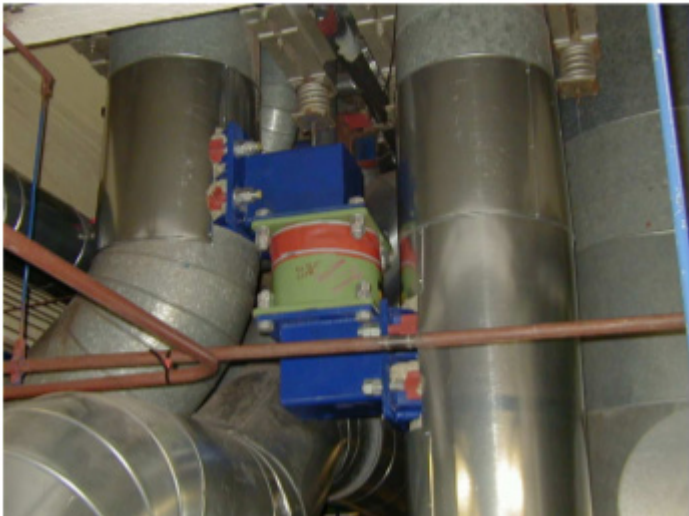
Figure 61: VD damper installed between to RA lines with different dynamic properties.
