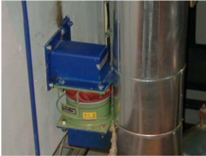
Figure 62: A VRD damper installed at RA10 line in Turbine Hall with the housing at the piping and the piston attached to the wall using a horizontal bracket.
