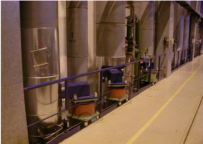
Figure 59: Three dampers installed in the Turbine hall
