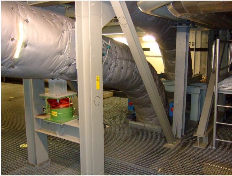
Figure 40: Installation example of viscous damper and supporting structures.
