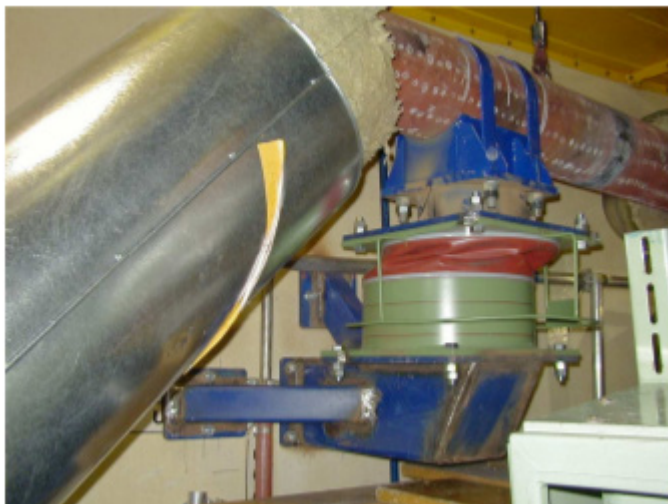
Figure 58: VES damper installed in Reactor Building LO2 at RL76. Damper's piston at the piping and housing fixed to the RB wall.
