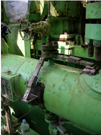
Figure 18: Damper link with Small Bore Fitting (SBF) bracing with glued saddle plates
