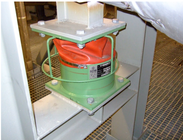
Figure 41: Installation example of viscous damper and supporting structures.
