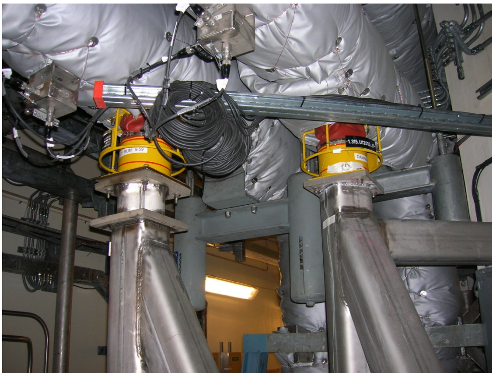
Figure 51 Viscous dampers mounted on condenser lines 1 and 2.
