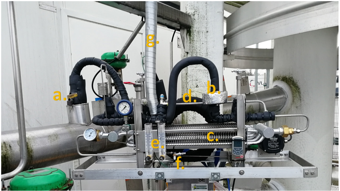
Fig. 3 Picture of the sampling system connected at the Stigs Center station. Parts of the system: a) Connection to the station pipe b) Insulated filter-holder c) Vaporizer for the particle section d) Heated vaporizer for the gas sampling e) Flow meters f) Gas sample outlet g) Boil-off "chimney".
