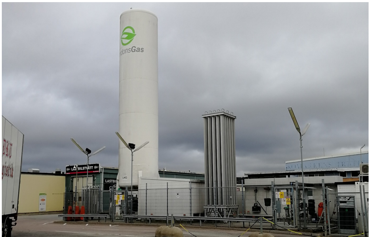
Fig. 2 Picture of the LNG/LBG refuelling station in Hisings Backa, Sweden, where the sampler was tested.
