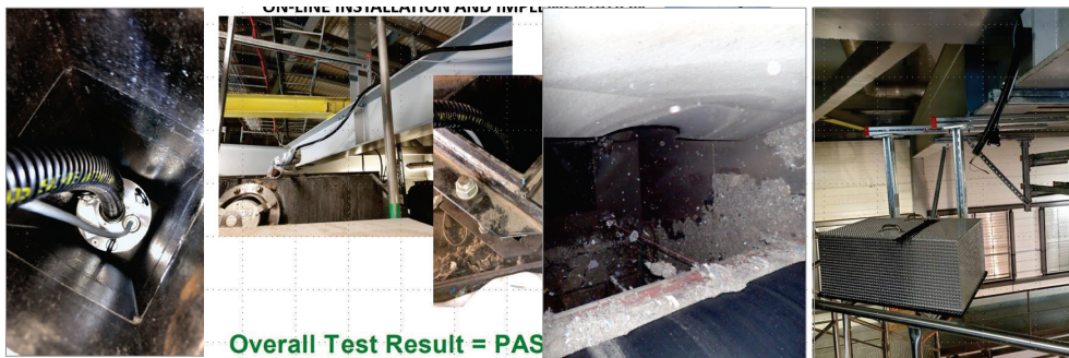
Figure 37: Details of NIRS head installation over the conveyor belt at Mälarenergi
