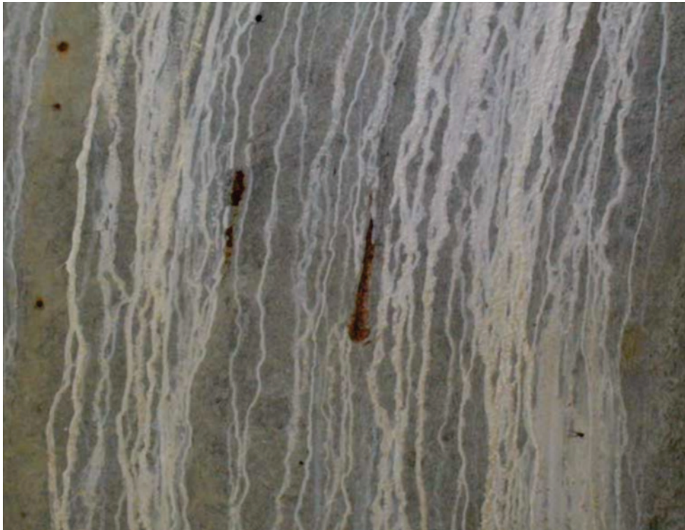
Figure 4. Calcite in cracks and visible corroded rebars [9].
