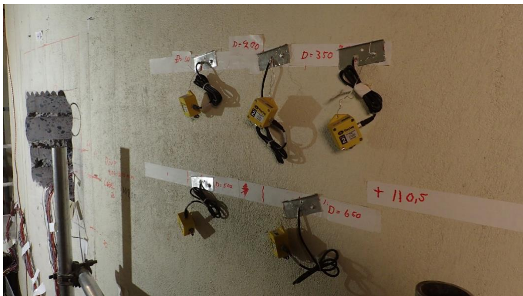
Figure 13 Installation of moisture measuring sensors on level 10,5.
