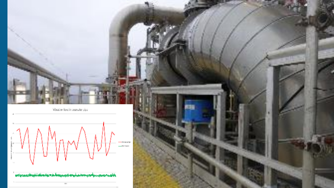
Produced water return
