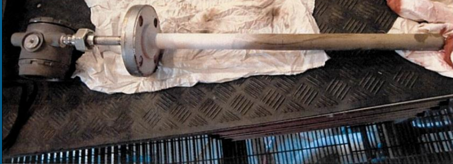
Thermowell with crack
