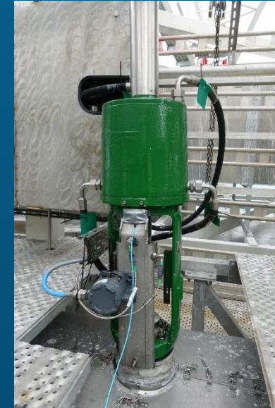
Anti surge valve
