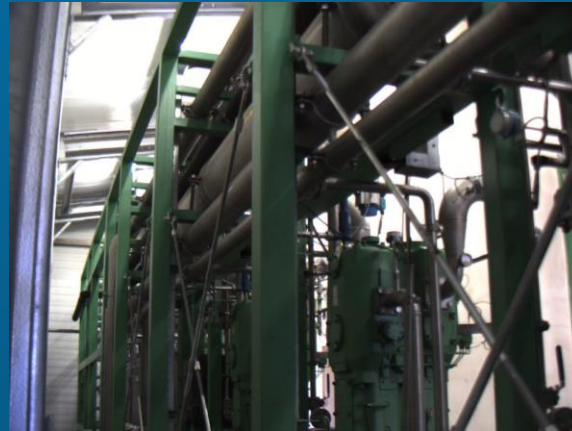
LF from compressor
