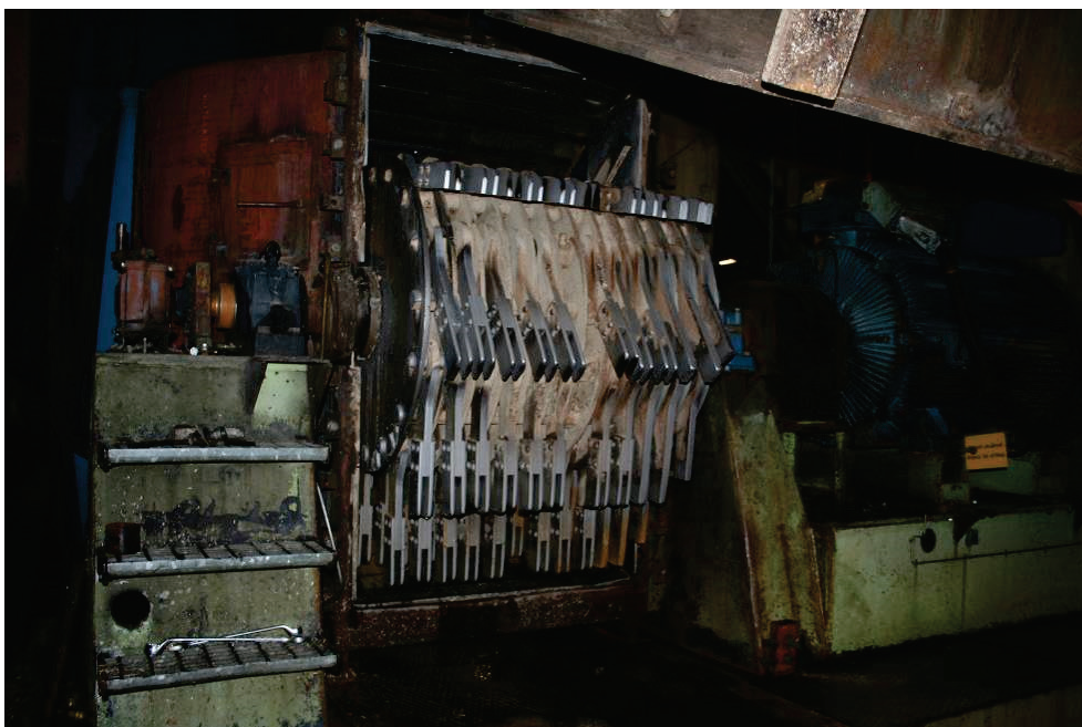
Figure 13. Hammer mill opened for inspection.
