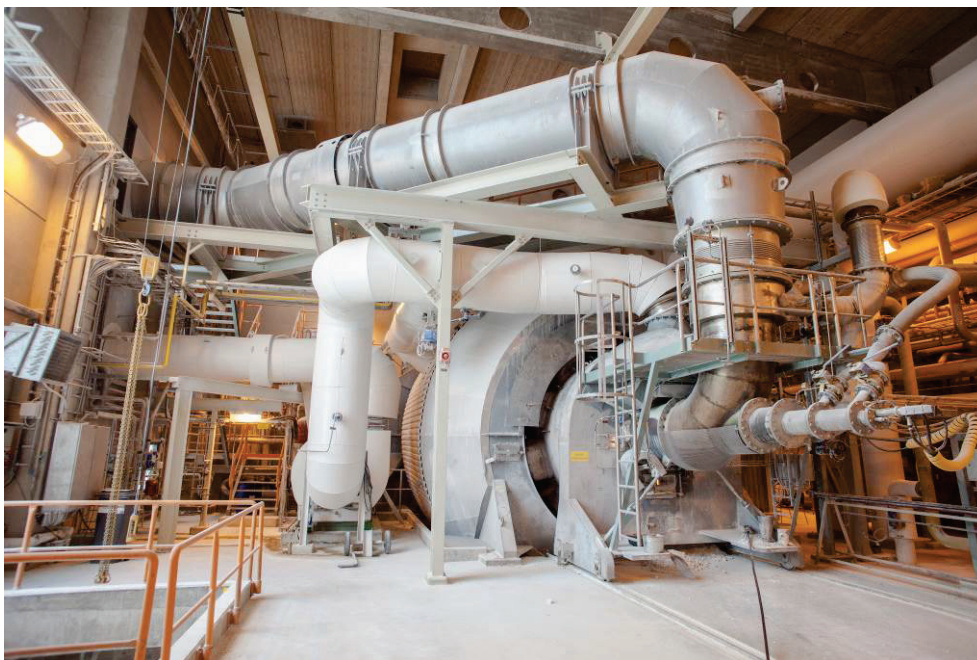
Figure 6. Multi-fuel burner used to fire gasified bark. (Source: ANDRITZ)
