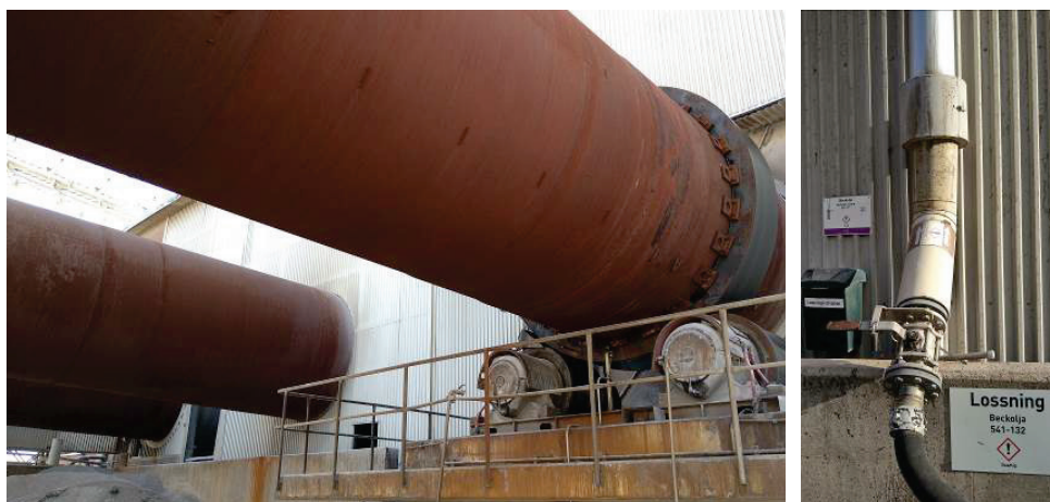
Figure 8. Discharge end of the three lime kilns in the Gävle mill (left) and the unloading station for tall oil pitch (right).
