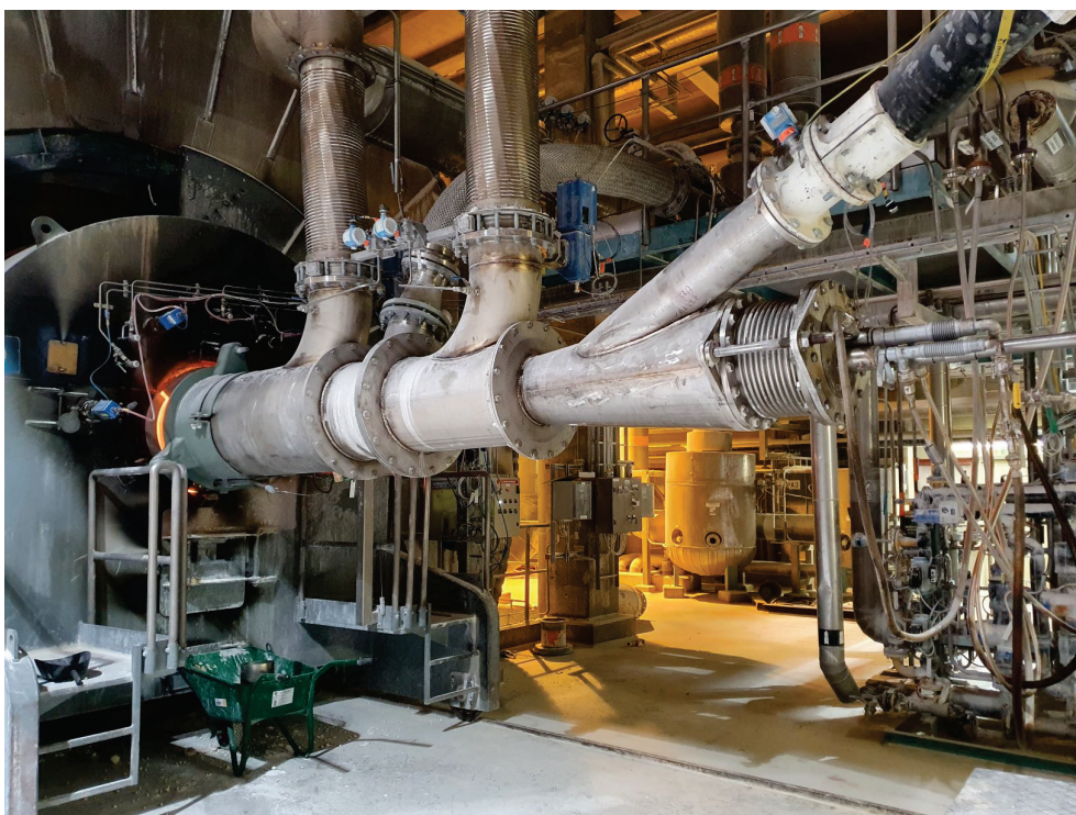
Figure 5. Combination burner (wood powder and methanol) at the Östrand mill.
