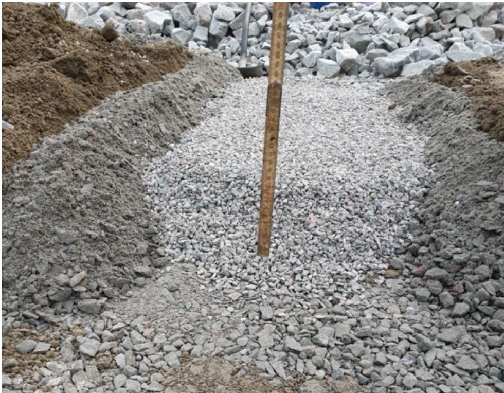
Figure 10 Defect 2 taken during construction (photo from Vattenfall)
