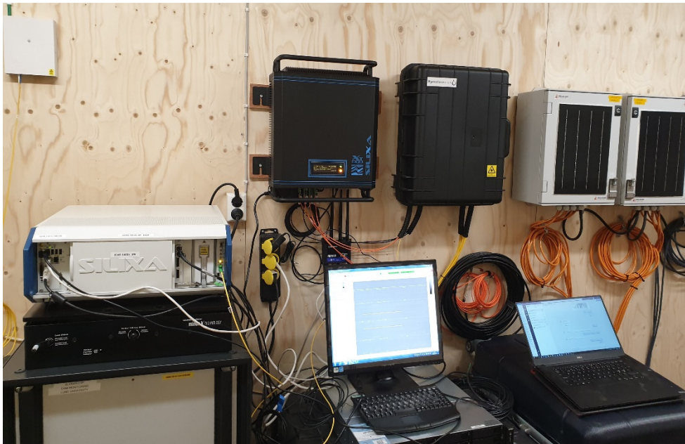
Figure 4 Monitoring unit for DAS and DTS, inside the monitoring container.
