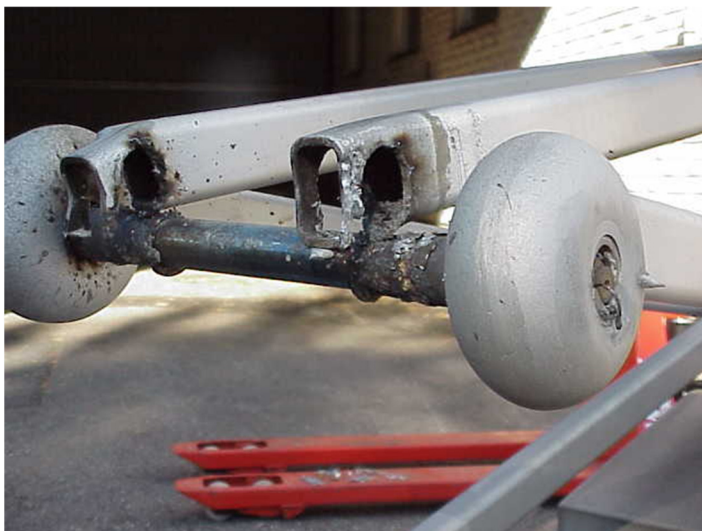
Figure 9 Close up photo of the overheated and broken disconnector in the substation at the west coast.
