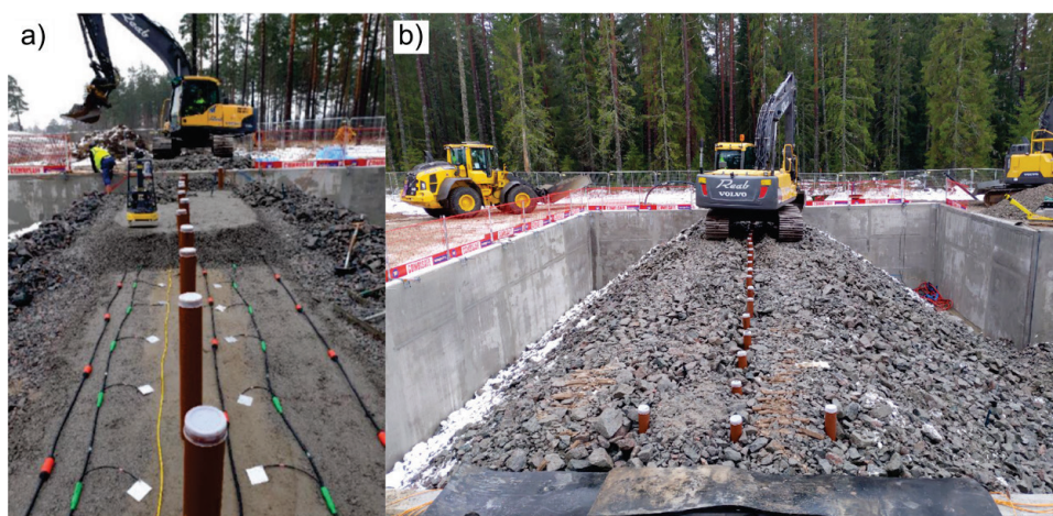
Figure 3. (a) Installation of geophysical equipment (hydrophones (red and black cable) and electrodes (green and black cable)) within the structure of the dam. Boreholes made of PVC casing are approximately 0.55 m deep from the top of the dam. (b) Last works on the crest of the dam before finishing the construction.
