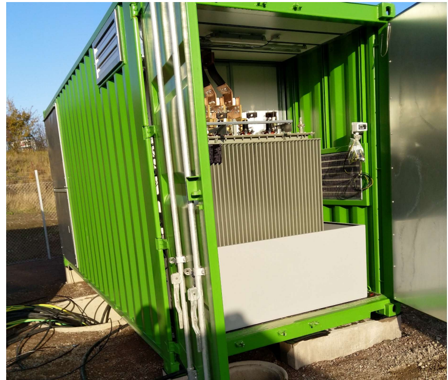
Transformer and inverter container
