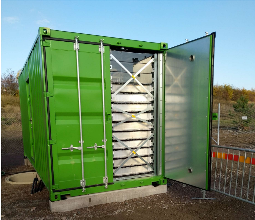
40 BMW EV car batteries in one container
