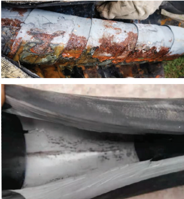
Figure 11 Examples of failure damages appeared at MV cable accessory interfaces due to multi-physical stresses combined with water ingress.
