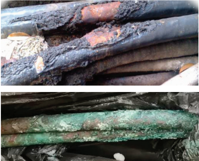
Figure 13 common damages found at cable body, top: third party damages; bottom: water damages.
