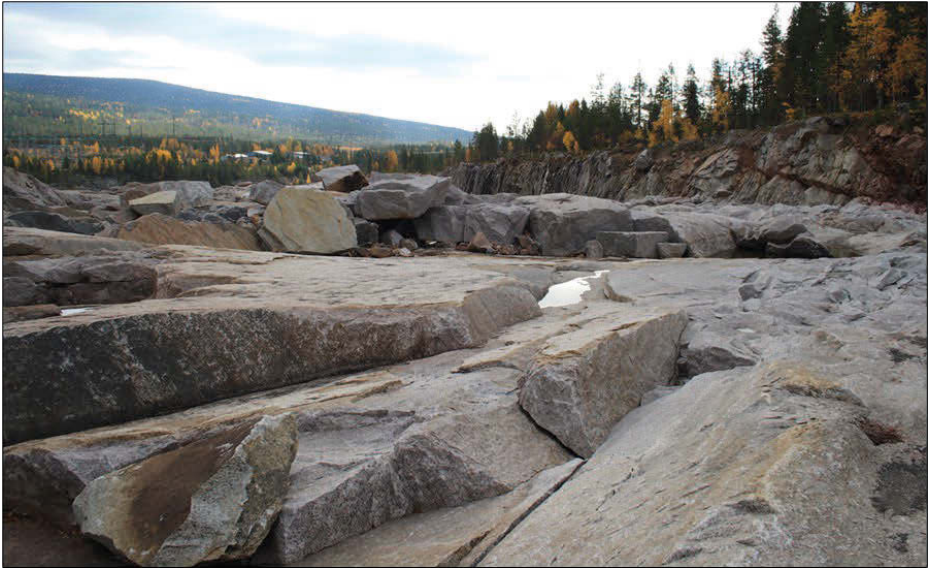
Figure 11. Dam 1 spillway block erosion.
