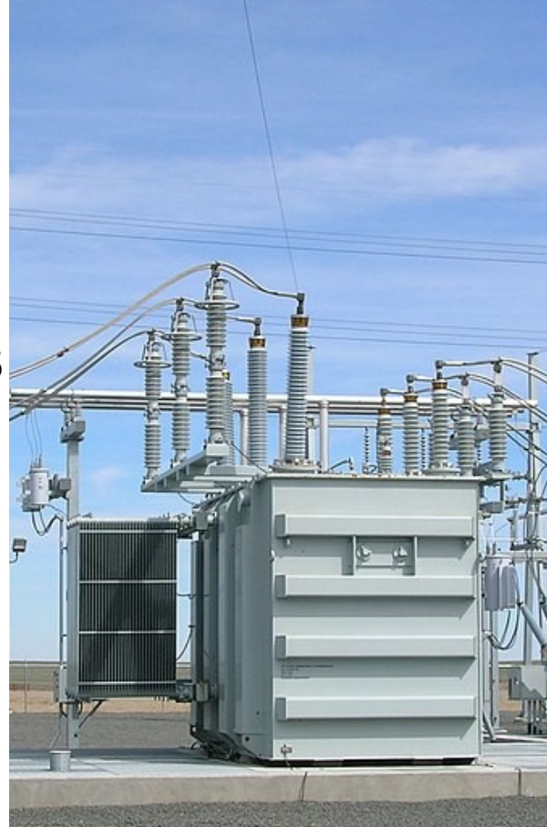
Transformers at substation near Denver International Airport, Colorado – Wikimedia commons
