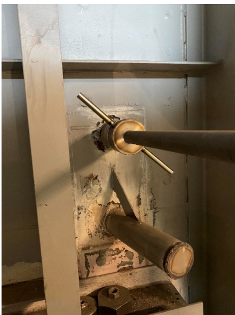
Figure 32 Installed probe in Mälarenergi P6 boiler system. The probe was mounted into the horizontal manifold duct just before the empty pass.
