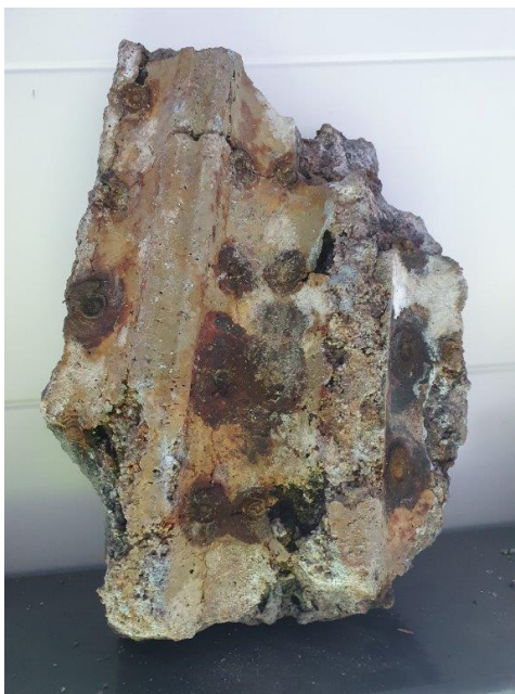
Figure 1 Examples of corroded studdings in a detached piece from P6 chamber roof.
