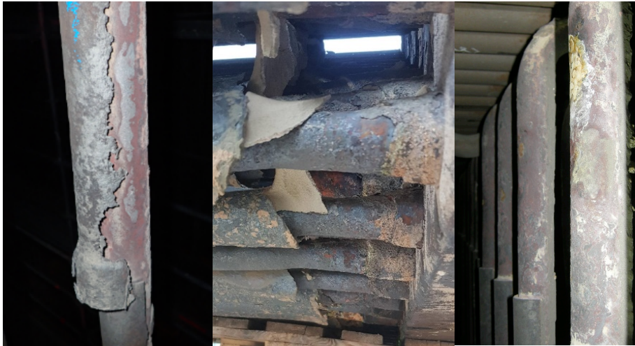
Figure 3 Corroded and eroded tubes with tube shield in P15 (left), SH3 in P14 (middle) and SH2 with ChlorOut additions in Jordbro.
