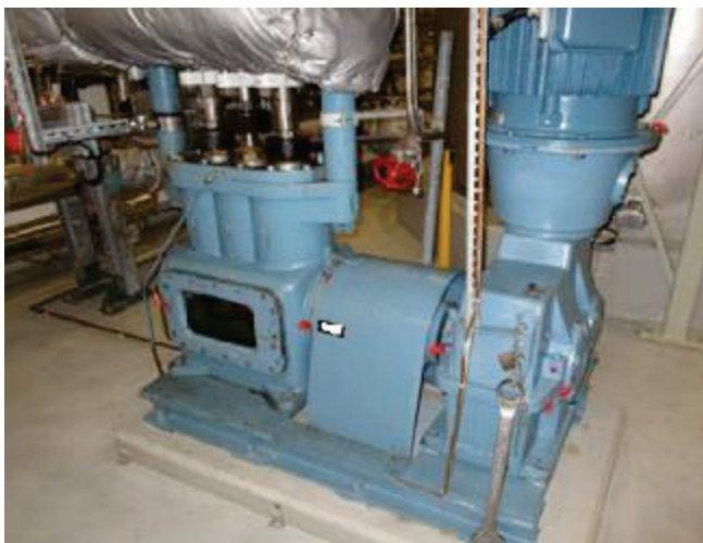
Figure 10: Example of piston pump at a BWR plant
