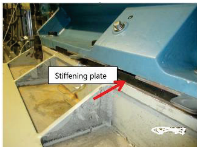
Figure 60: Motor mounted with extra steel stiffening plate mounted with bolts and shims on each side of the motor frame
