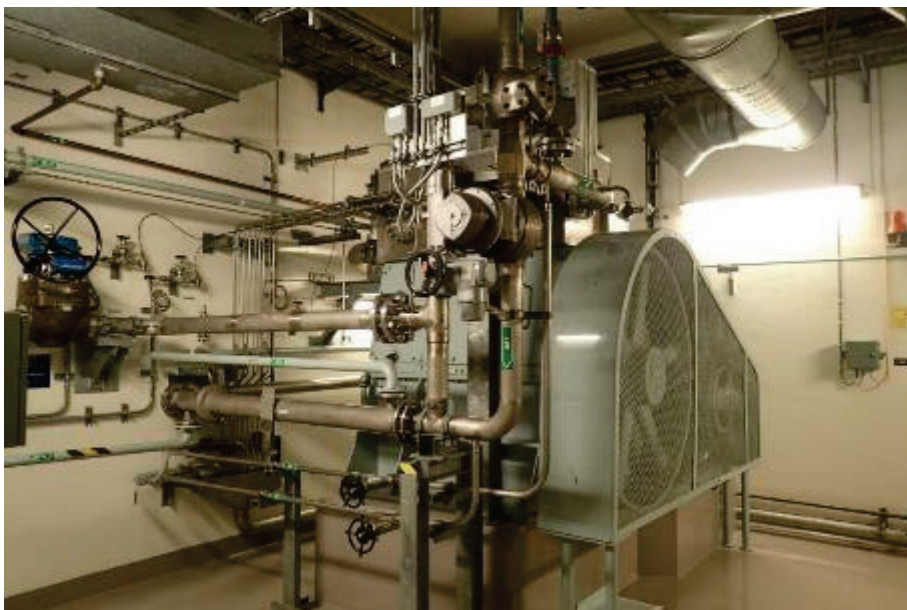
Figure 31: Plunger pump on a high-pressure safety system.
