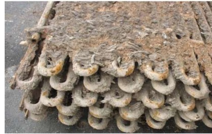
Fig. 2.2. Deposit formation on a superheater used in a grate fired boiler during combustion of waste wood. Kassman, H. (2012). Strategies to reduce gaseous KCl and chlorine in deposits during combustion of biomass in fluidised bed boilers.
