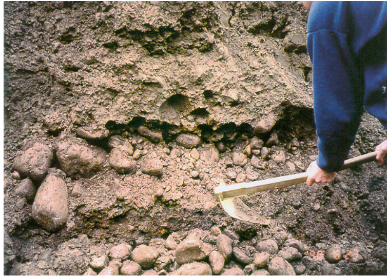
Figure 3 A cross-section of the dam at Lövön power plant during a dam reconstruction 1998. At the centre of the photographed region, the soil consists only of larger grains. Fines have been lost due to erosion. (Photo from Gräninge AB.)
