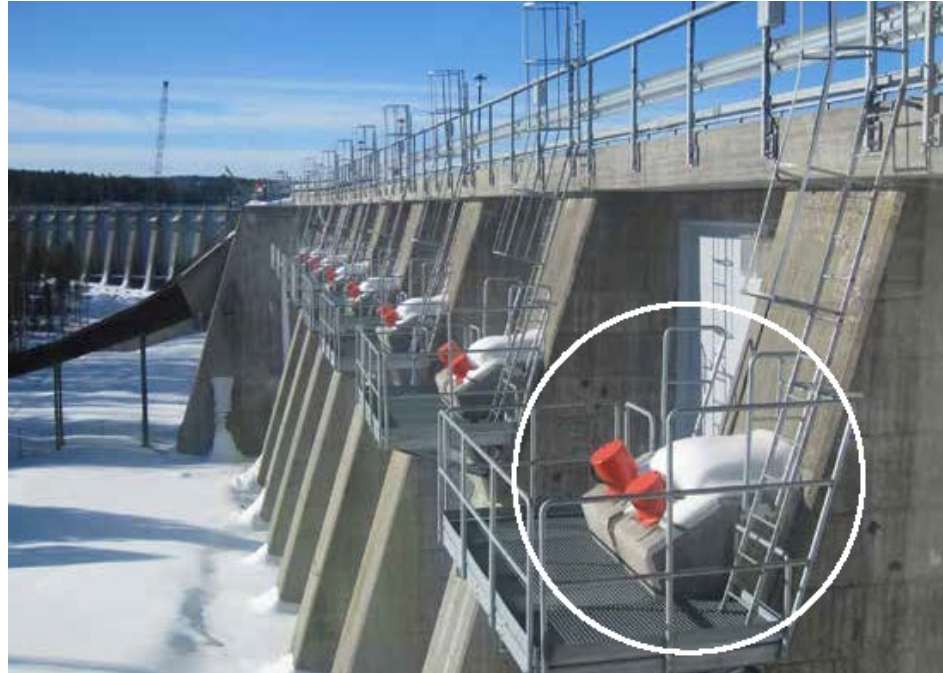
Example of stability enhancing measures, pre-stressed anchor cables at Storfinnforsen buttress dam (Photo Svenska Kraftnät)
