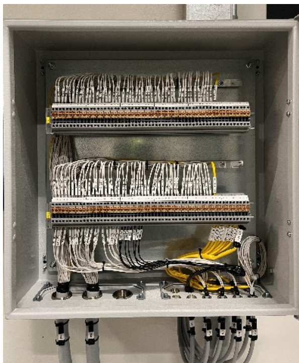
Figure 10 – Test Location 8 – Wiring Junction Box (ZHD.102)
