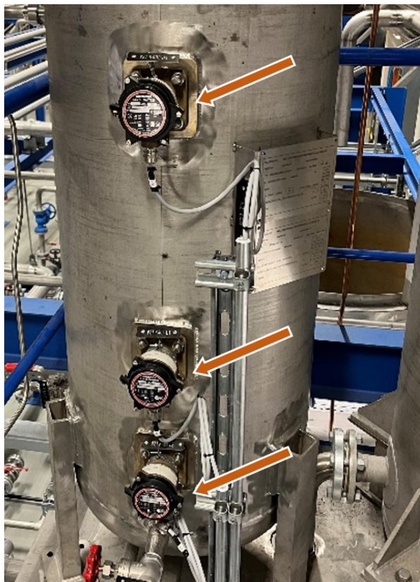
Figure 8 – Test Location 6 – Mobrey S01DB/84 Level Switch (Sensors 921K403, 921K404, and 921K405)
