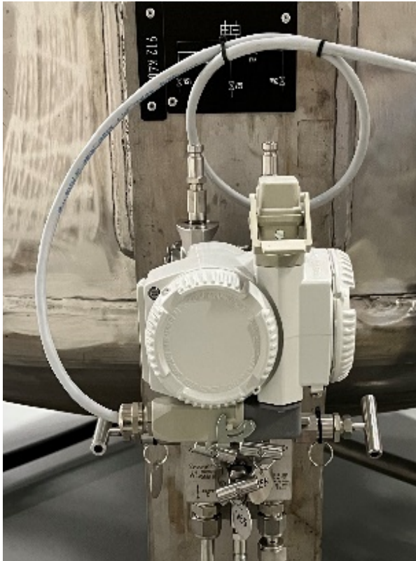
Figure 5 - Test location 3 (Sensor 912K401) – ABB 265DS Level Transmitter
