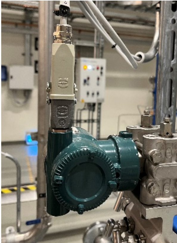
Figure 3 - Test location 1 (Sensor 912K202) – Yokogawa EJX110A Differential Pressure Transmitter
