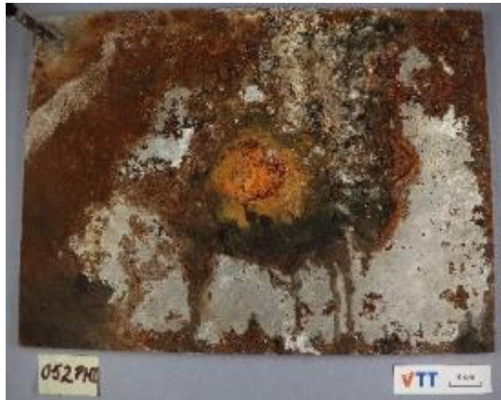
Bild från: M. Nilsson et al., "Non-destructive evaluation of corrosion in steel liner plates embedded in concrete using nonlinear ultrasonics," Construction and Building Materials , vol. 408, p. 133691, 2023. doi:10.1016/j.conbuildmat.2023.133691
