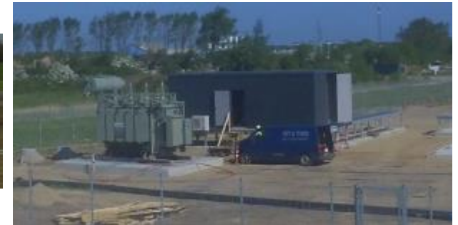
Transformer and electrical building
