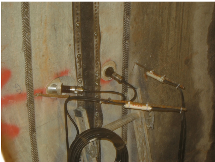
Figure 4—8 Joint meters used to measure the relative displacement between concrete and rock, Malm (2015).
