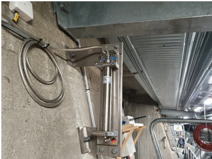
Figure 4—5 Tilt sensor installed near the crest of a concrete buttress dam.
