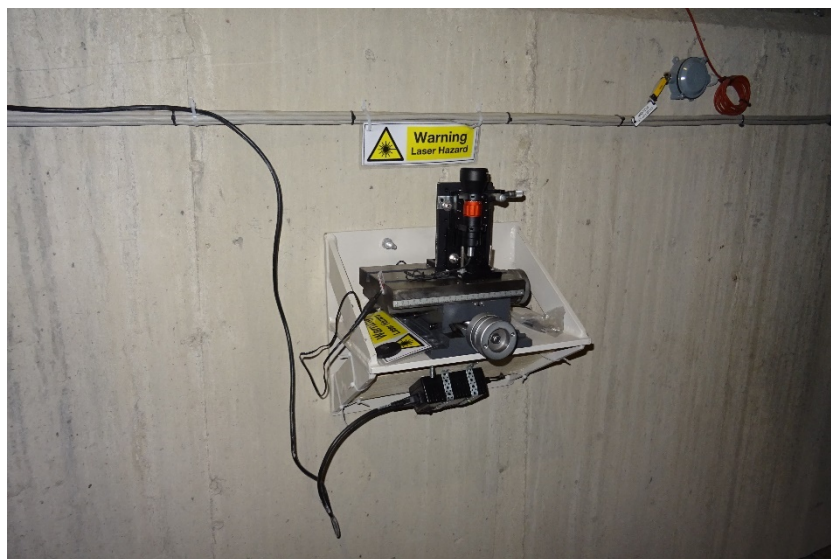
Figure 6—5 Laser mounted near the base on a Swedish concrete dam
