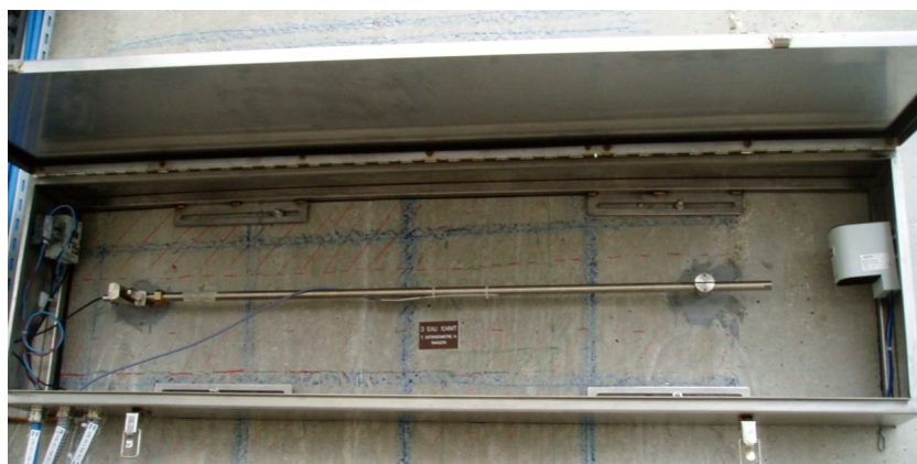
Figure 4—11 Surface strain meter installed on the outside of a containment wall. The displacement sensor is left side of the 1 \text{ m} invar bar, A. Simon et. Al (2013).
